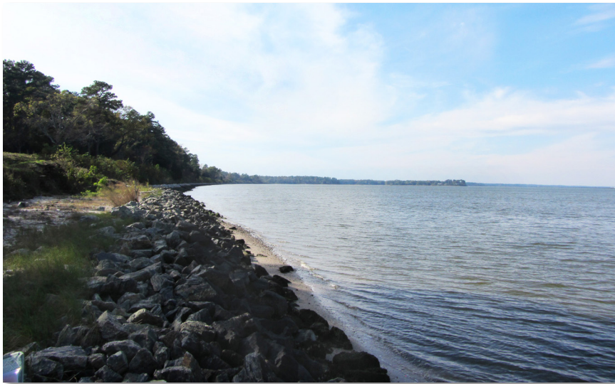
Figure 10. Revetment at Bellfield Straight along the York River (#83 Figure 9). View is to the west.
