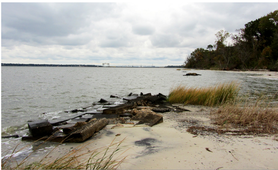
Figure 11. NPS broken concrete breakwaters along the York River (#87–91 Figure 9). View is to the southeast.
