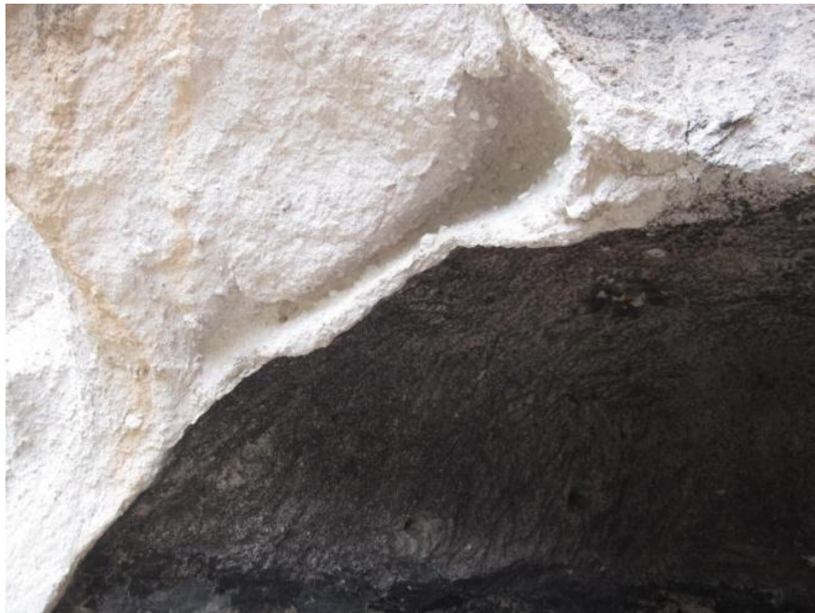
FIGURE 6. SAGGING OF SOOTED CEILING AT A-GROUP.
