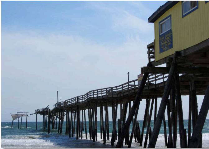
Figure 17. The Frisco Pier has been extensively damaged by storms and was closed in 2009 (#32 Figure 14) (image by Kate Dallas).
