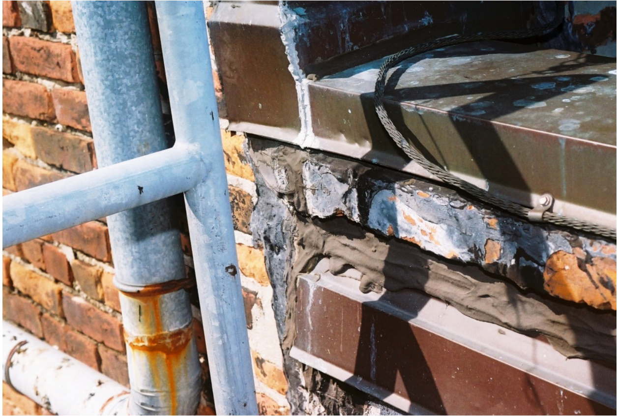
Photograph 22. This photo shows some of the upper and lower flashing at the edge of the building, which allows the American cockroaches to enter the underside of the roof. Neighborhood cockroaches have found this area to be a safe haven during the day.
