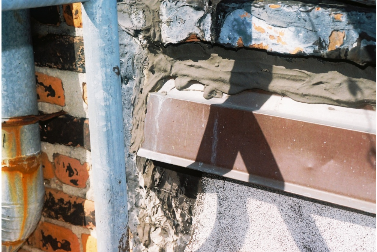
Photograph 24. This photo shows the lower flashing, which may also be acting as a highway for the cockroaches into the building. All of this flashing needs to be sealed.
