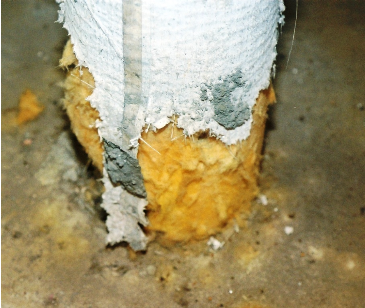
Photograph 11. American cockroach feeding on pipe insulation.
