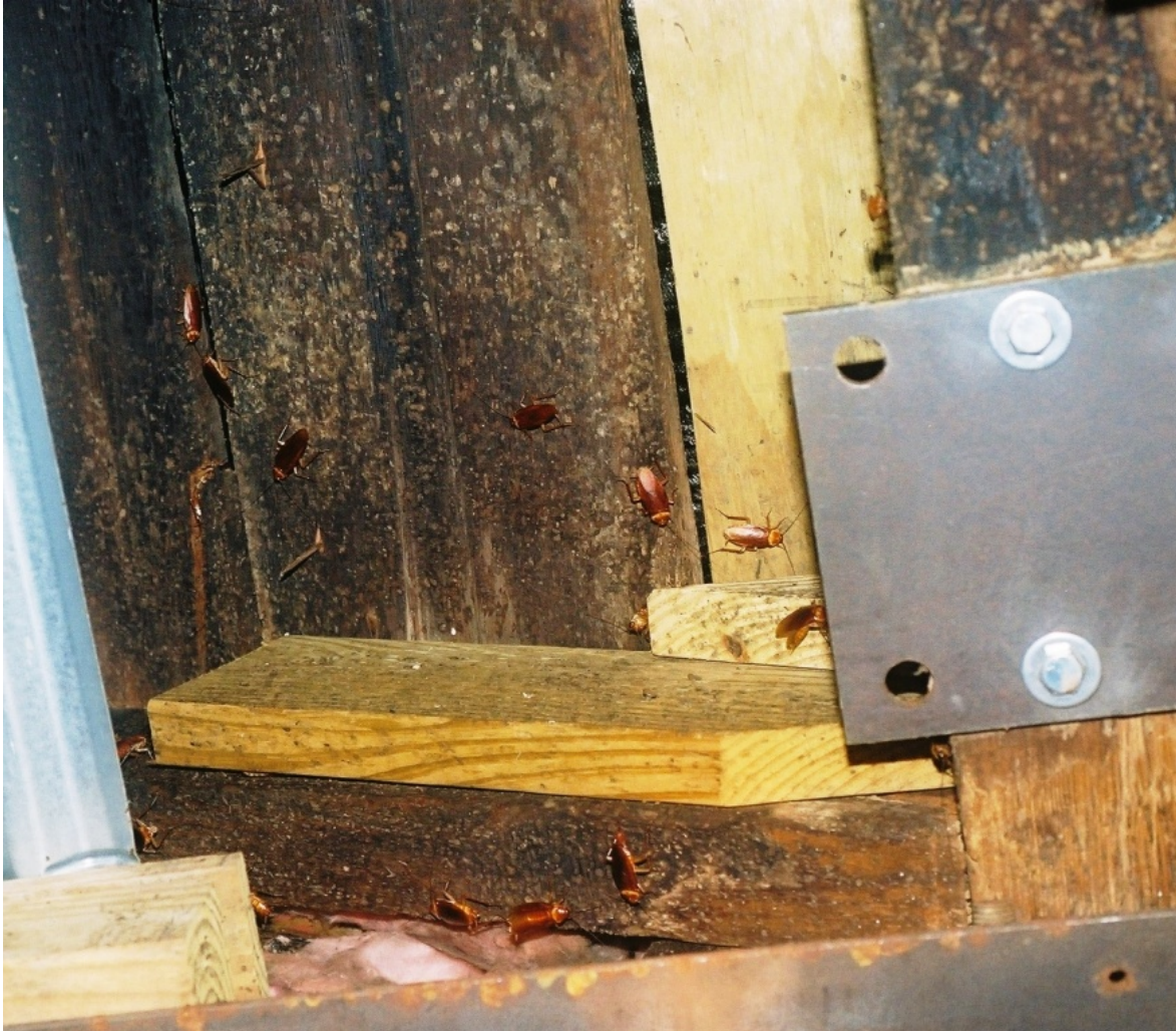
Photograph 17. Quite a few American cockroaches can be seen in this photo taken above the false ceiling in the hallway of Building 3 at the junction with Building 2. All appear to be adults with full wing covers. This necessarily means they are walking into the building from outdoors. If nymphs were found in this grouping, it would mean this was an in-house population. Adult cockroaches roam the streets and alleys at night looking for food. During the day, they return to this safe resting spot, producing their pungent odor.
