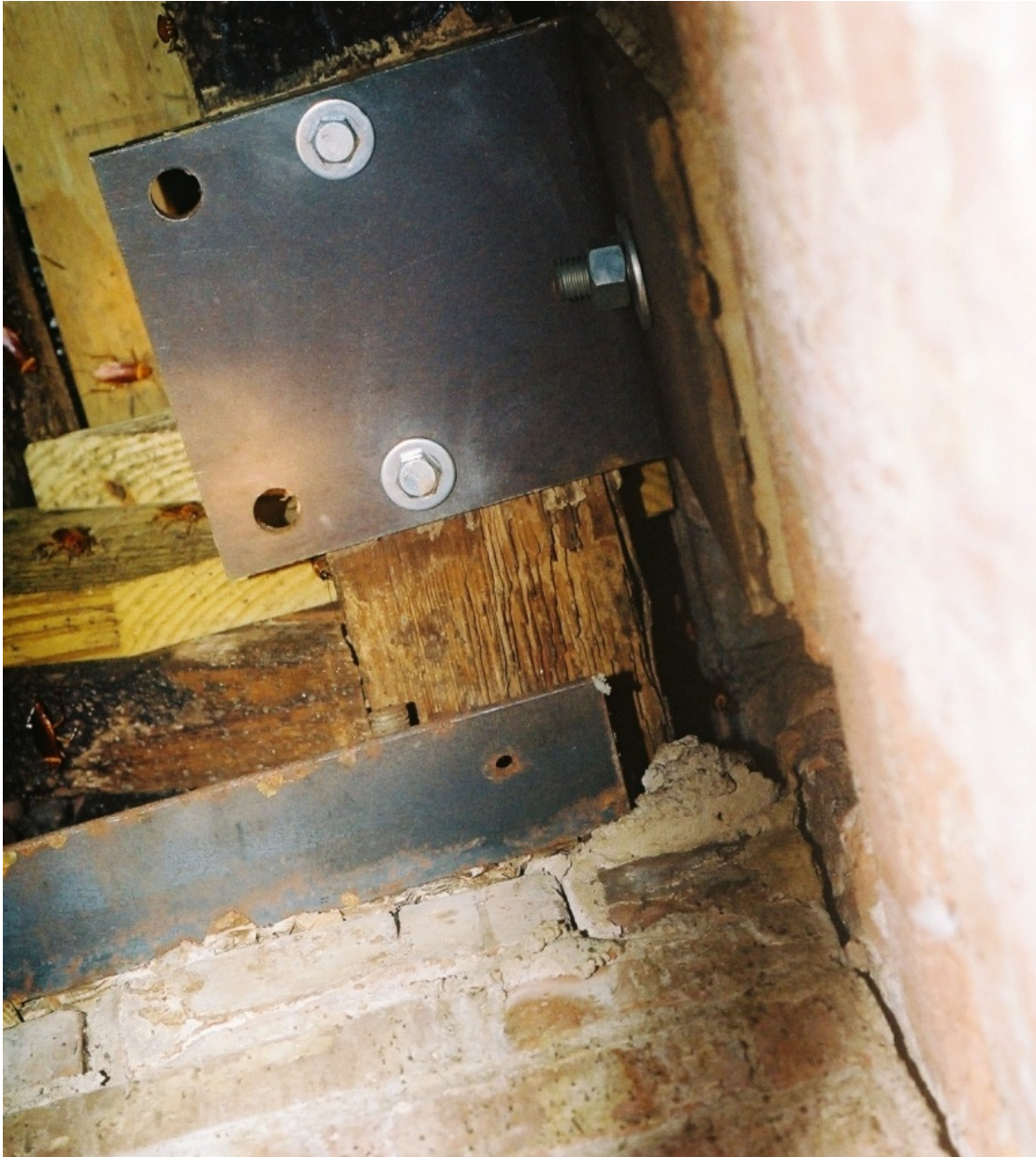
Photograph 18. This photo shows the gap between the French Quarter Visitor Center interior brick column and the exterior brick wall. Although it is difficult to see in this photo, there are several American cockroaches resting in this gap. Dark stains can also be seen where the cockroaches routinely venture down from their resting place into the building at night. This infestation has been present for years.
