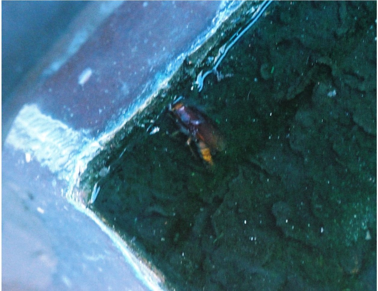
Photograph 26. Dead American cockroaches in the standing water of the gutter immediately adjacent to the flashing highways into the building.
