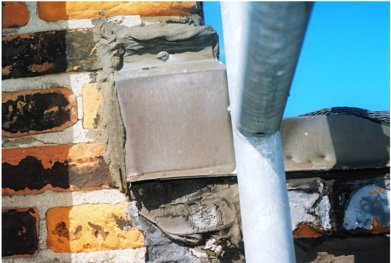
Photograph 23. I consider this piece of flashing on the corner where the abandoned building meets the wall of Building 3 to be a major highway for the American cockroaches to gain access to the underside of the roof.
