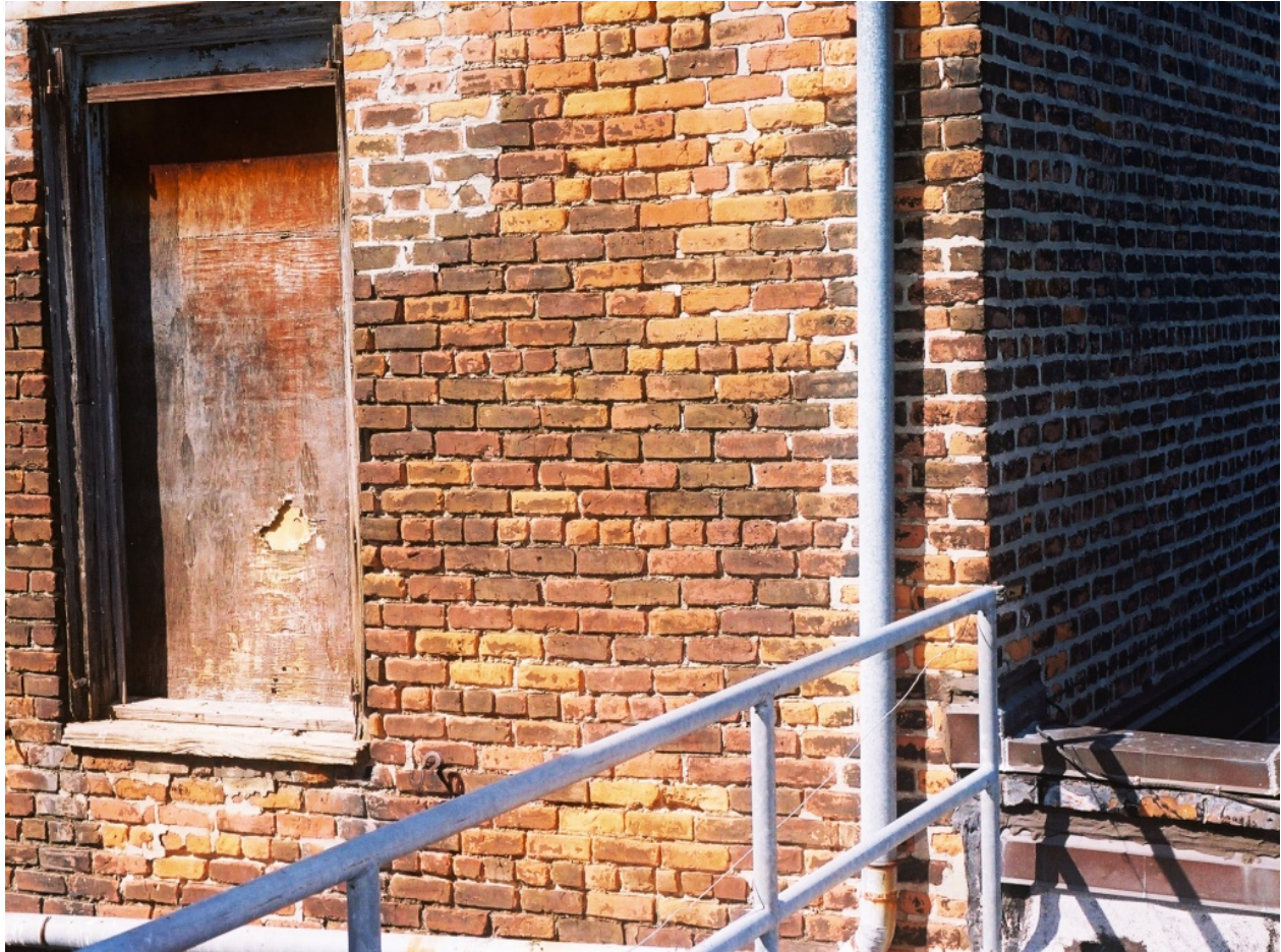
Photograph 20. This photo shows the abandoned building adjacent to the French Quarter Visitor Center where it abuts the junction between Buildings 2 and 3. The flashing shown in the lower right of the photo is the area where the American cockroaches enter the Visitor Center at the parapet/peaked roof.
