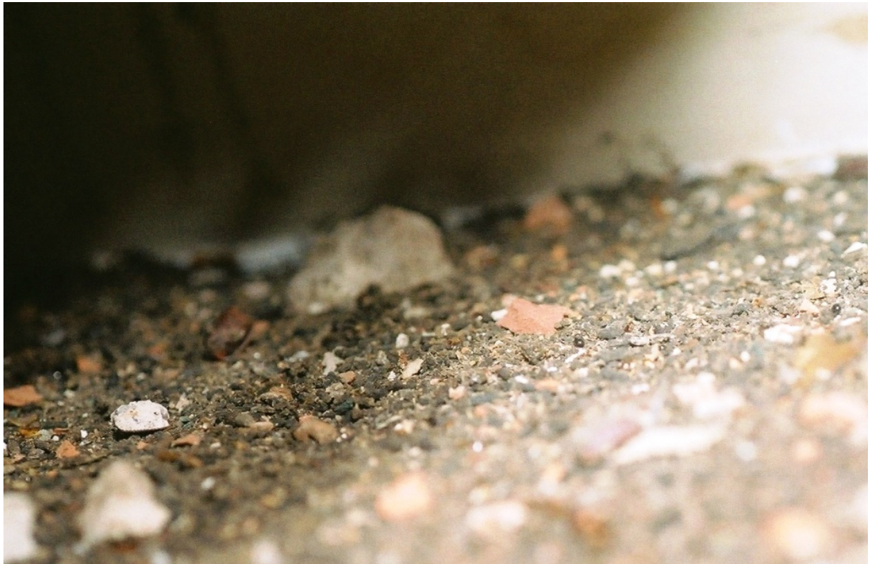
Photograph 16. American cockroach droppings accumulated on a ceiling tile above the hallway between Buildings 2 and 3 on the second floor. American cockroaches excrete a pelletized dropping, which looks similar to a mouse dropping. It can be differentiated from a mouse dropping by its blunt ends and ridges running the length of the dropping. They are usually black in color. Some can be clearly seen in the center left of this photograph, along with debris from the old brick wall.
