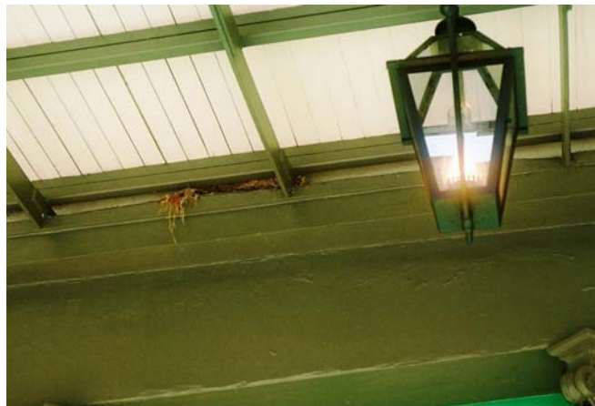
Photograph 6. An English sparrow nest above the green doors.
