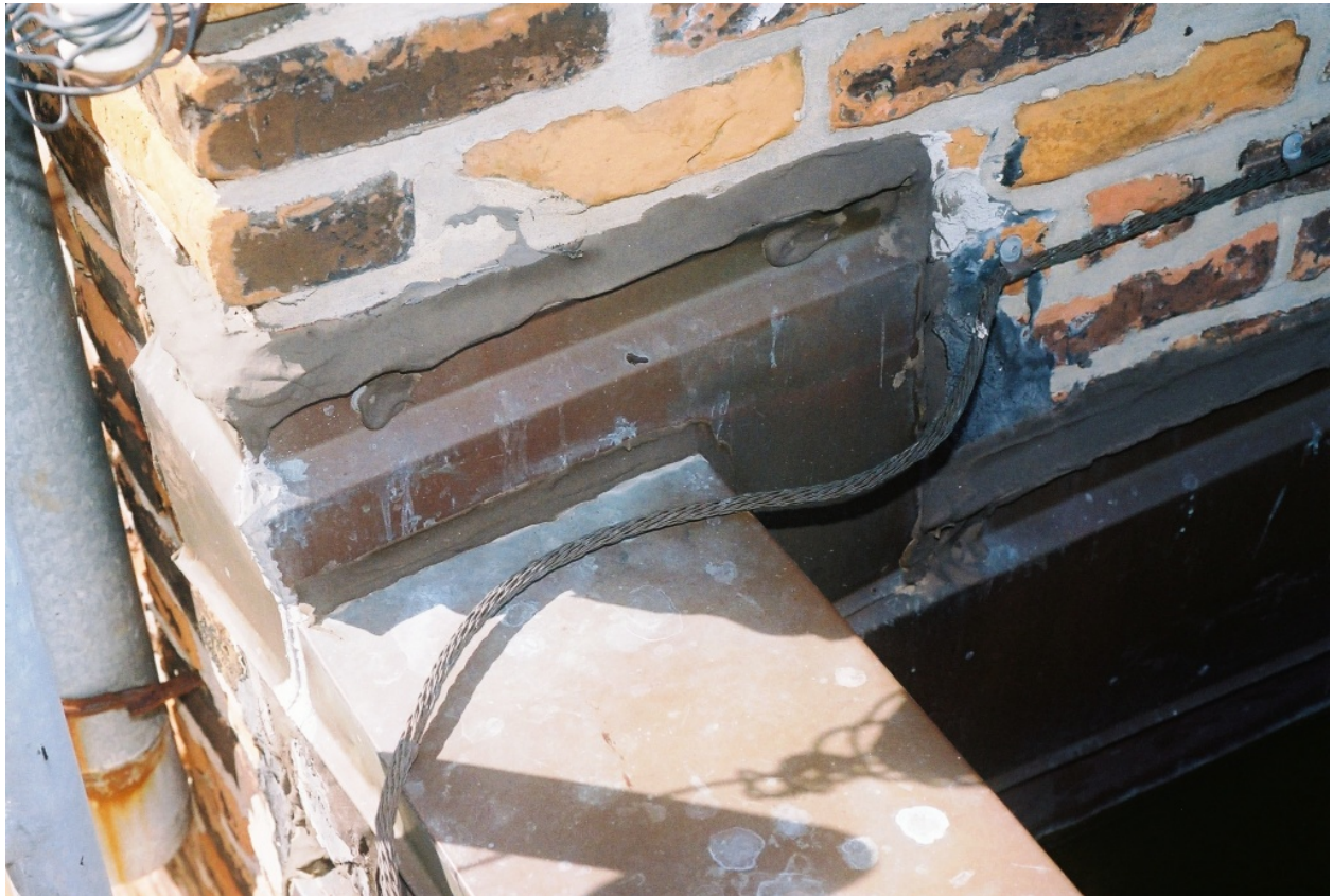
Photograph 25. Once the cockroaches climb up under the flashing, they can easily crawl in the gap behind the flashing and down into the underside of the roof. All flashing on both sides of this parapet/peaked roof must be thoroughly sealed.
