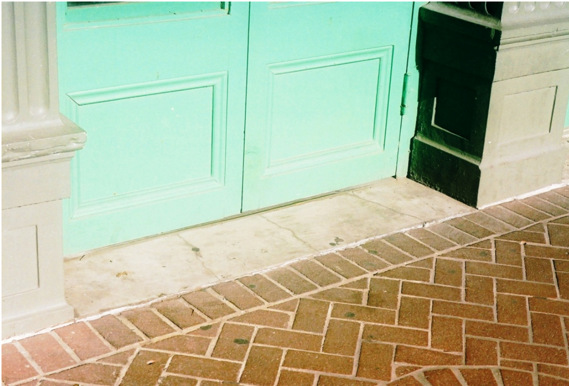
Photograph 4. Substantial gaps beneath the double, wooden front doors.
