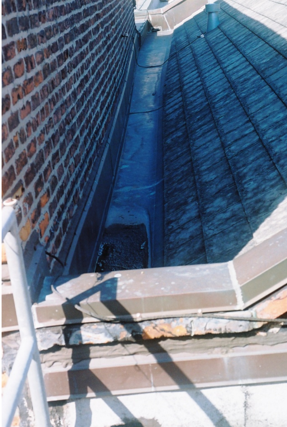
Photograph 21. The flashing on the parapet portion of the peaked roof of Building 3 allows the American cockroaches to climb up under the flashing and access the underside of the roof. Aerosol foam caulking or polyurethane caulking can be used to seal these cockroach highways after the populations have been substantially reduced on the interior.
