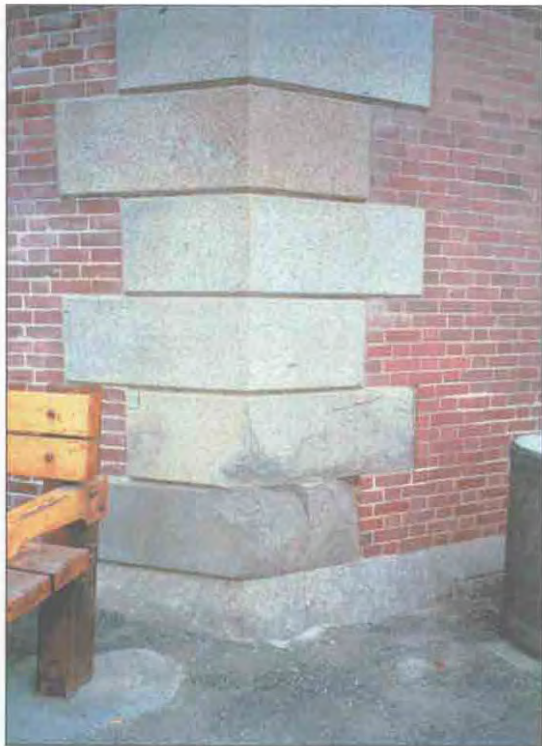
Condition Photo 7: East Bastion—East Hank; impact damage at granite quoins and base. (Courtesy of ARG, 2003)
