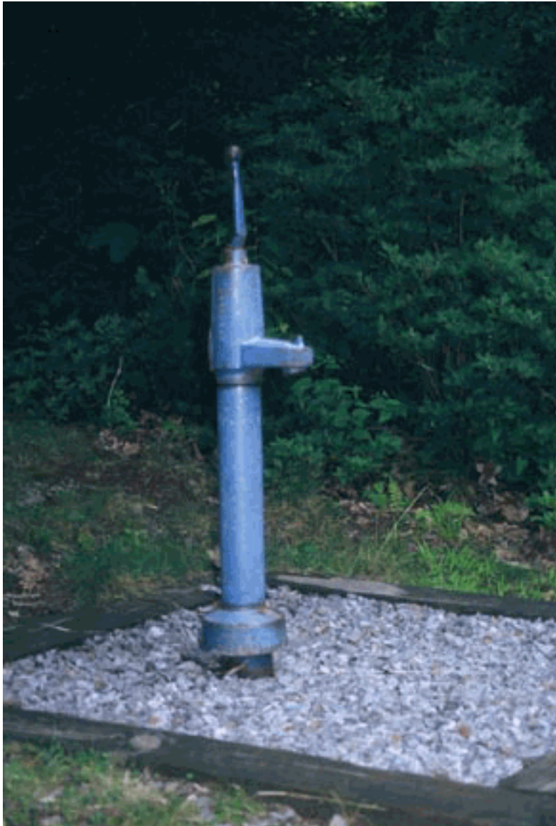
Figure 16: Typical water pump (NPS).
