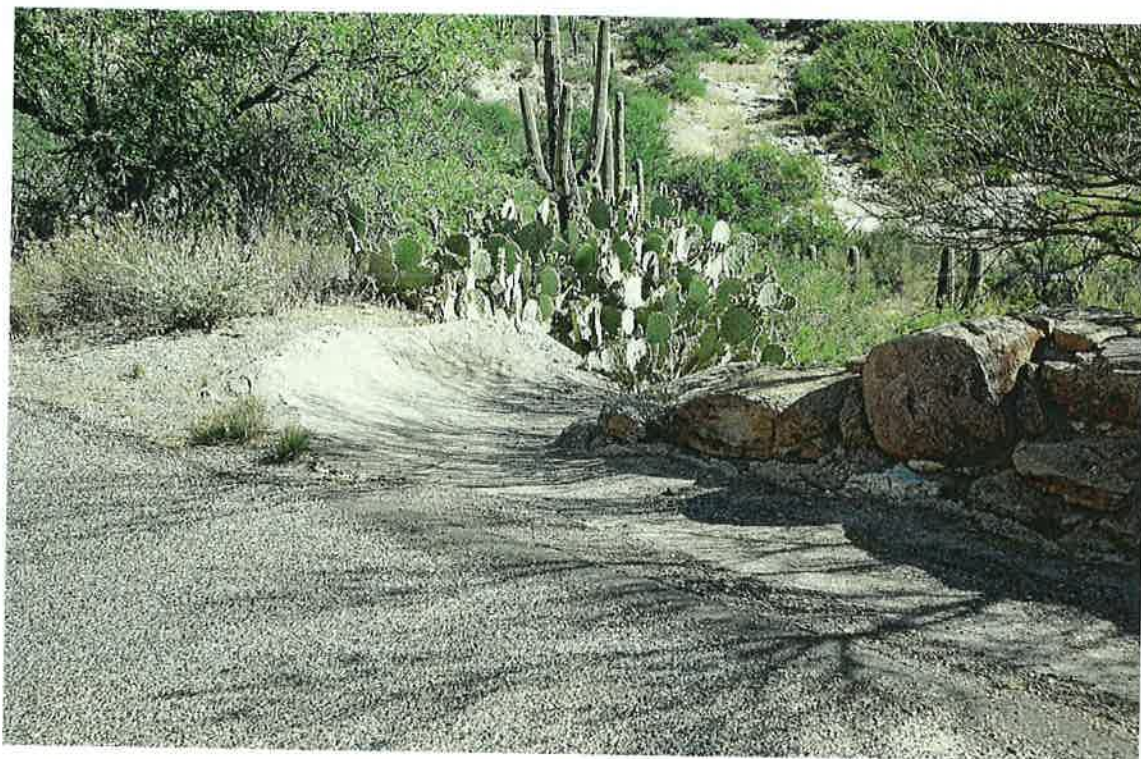
FIGURE 27. EXAMPLE OF CEMENT DRAINAGE, VIEW FROM ROADBED
