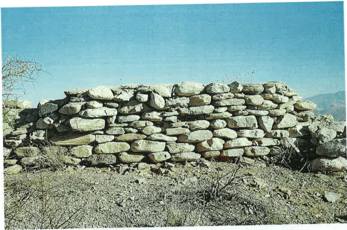
FIGURE 19. BACK SIDE (SOUTH SIDE) OF THE WALL (NOTE LACK OF MORTAR)
