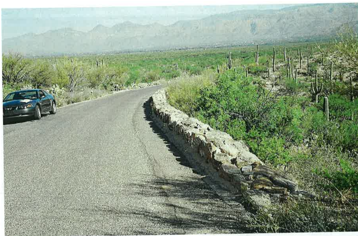
FIGURE 22. SEGMENT 1 – VIEW ALONG ROADBED LOOKING DOWNHILL (NOTE: CEMENT CHANNEL AGAINST RETAINING WALL)
