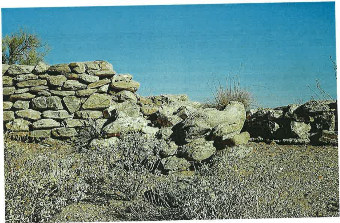
FIGURE 20. PORTION OF THE BACK SIDE THAT HAS COLLAPSED / TUMBLED (EASTERN END)
