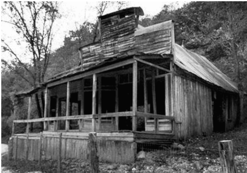
Taylor-Medley General Store before reaching current level of deterioration (NPS undated)
