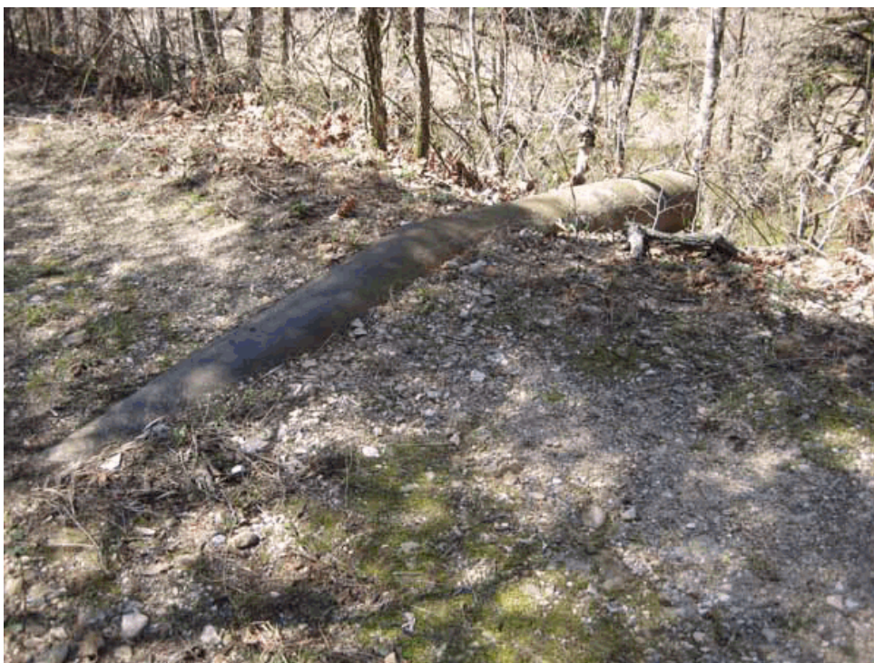
Steel piping at Monte Cristo Mine site (NPS 3/2011)
