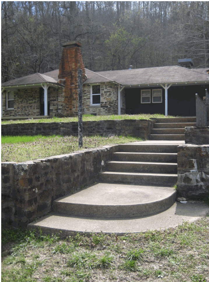
Current condition of the concrete walk and stairs (NPS, 2009).
