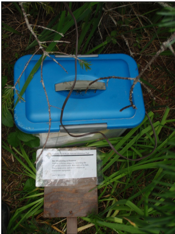
Figure18. Gel cell battery in housing.
