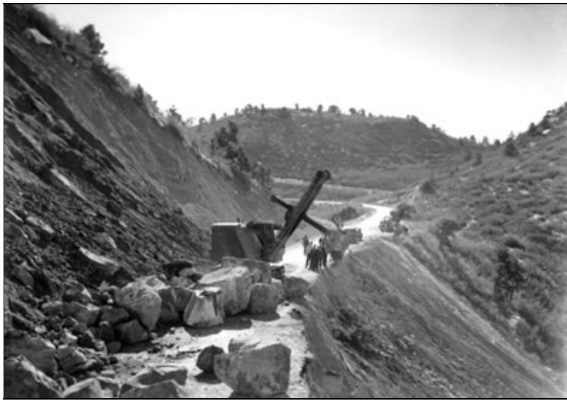
The Mancos shale under Knife Edge Road tended to slide, which did little to bolster tourists' confidence. Fortunately, this slide came in November 1941, after the park had closed for the season. (Courtesy: Mesa Verde National Park)
