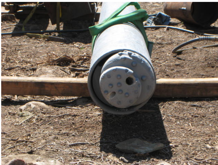
Figure 4. Photograph of under-reaming bit wedged in shoe at end of nominal 10-inch casing after pulling casing, drill stem, air hammer, and bit on May 11, 2012 at well site 1 east of sewage lagoons, Great Basin National Park, White Pine, County, Nevada.
