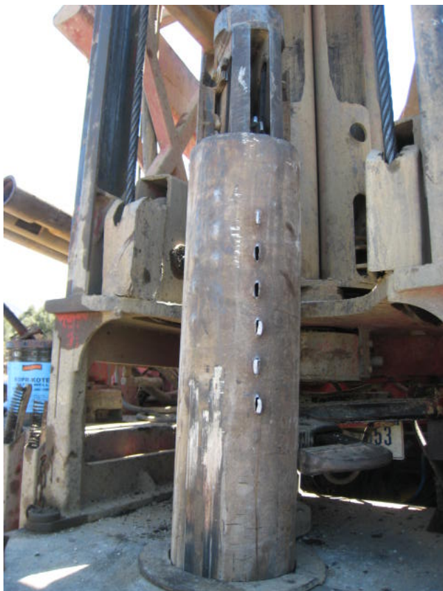
Figure 6. Photograph of nominal 8-inch casing showing perforations following a test on June 3, 2012 at well site 1 east of sewage lagoons, Great Basin National Park, White Pine County, Nevada.
