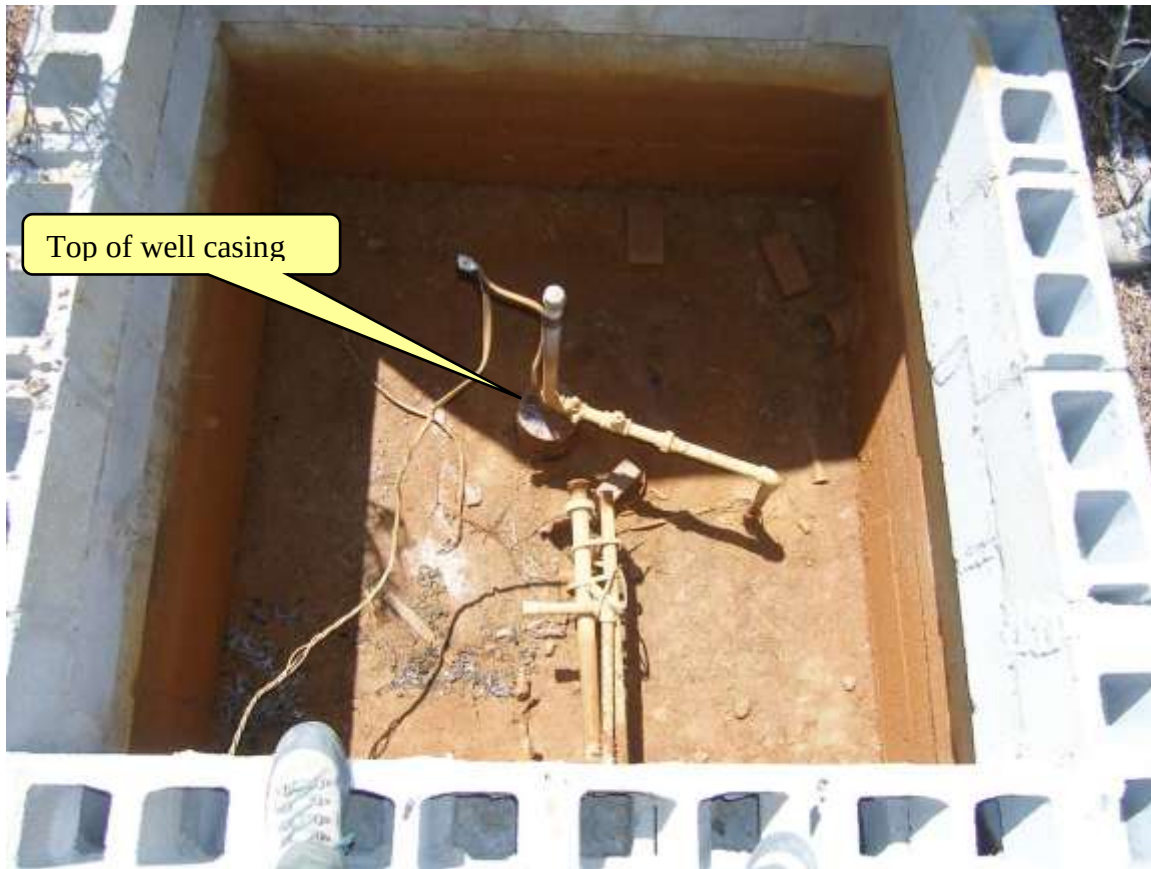
Figure 2. Well pit. The staining on the walls shows that water in the pit is frequently above the top of the well casing, creating the potential for contamination of the well.
