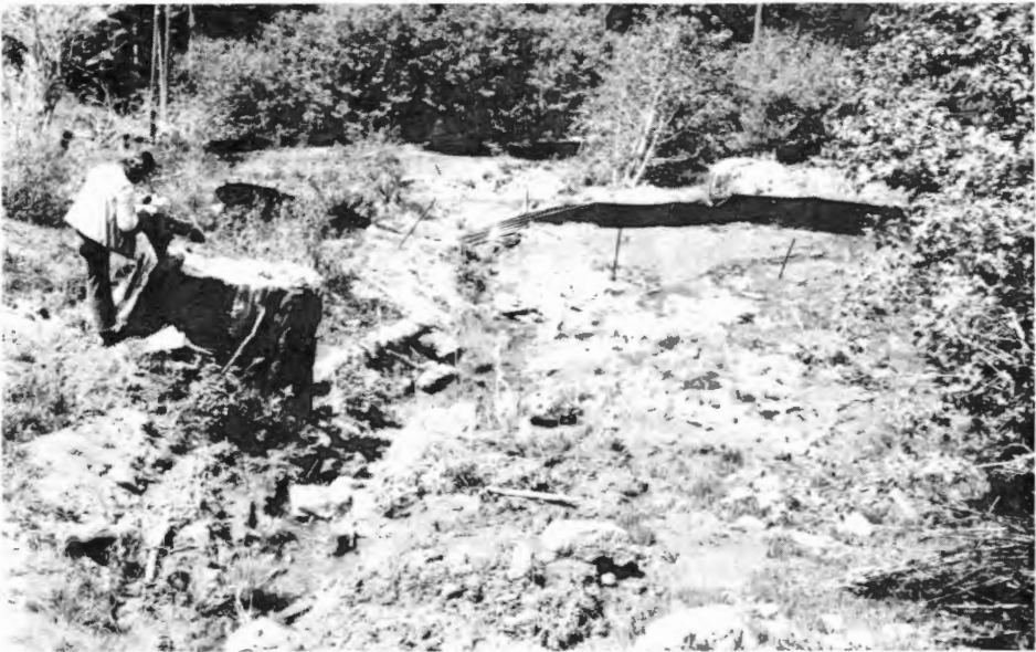
The view downstream with Check Dam No. 3 in the foreground and No. 2 in the distance. Dam No. 3 also has failed as a result of the landslide and mudflow above. The same potentials for failure exist here as exist at Check Dam #2.
