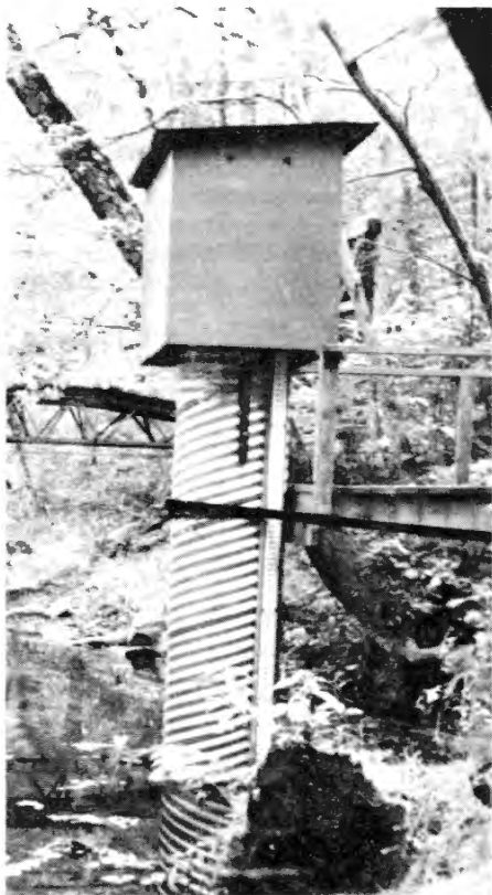
One of the four gaging stations along the Quantico Creek in Prince William Forrest Park. It houses water level monitoring equipment and an automatic water sampler.
