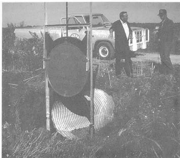
Landowners can receive financial assistance for water control structures such as this one to manage water levels in their wetlands.
