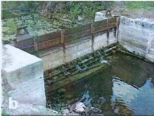
Photo 2-7. Photo of Gate 5 at Deep Lake under open (a) and close (b) conditions.
