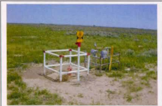
15. El Paso natural gas pipeline meter located on subject property's western one-half and immediately north of Road W.
