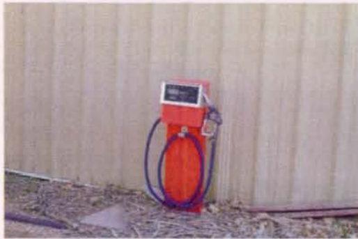
3. Abandoned gasoline dispenser located on the west side of the metal shed (see previous).
