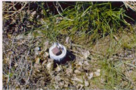
4. Refueling cap to an abandoned 1,000-gallon gasoline UST located on the north side of the metal shed (see Photo #2).
