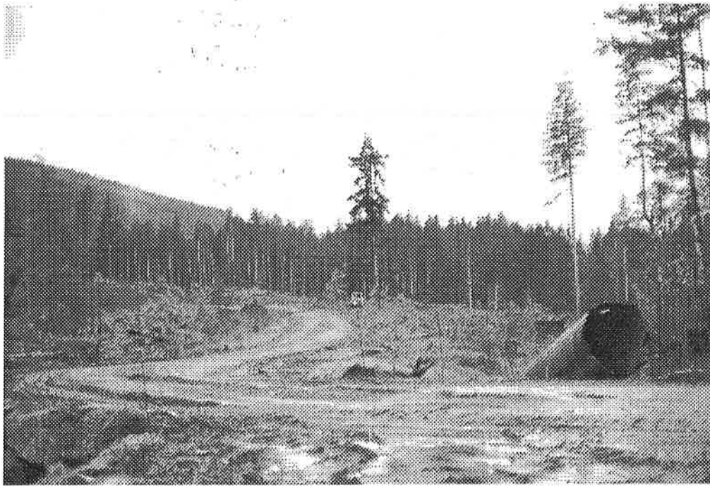
W2-10 Distal end of segment 11, condition class C
