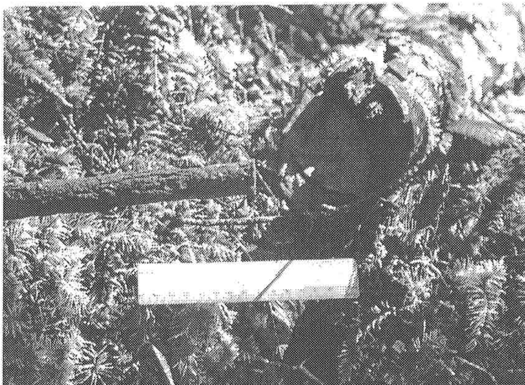
W2-5 Drift pin in timber, showing spalling. Sol Duc bridge site, segment 13
