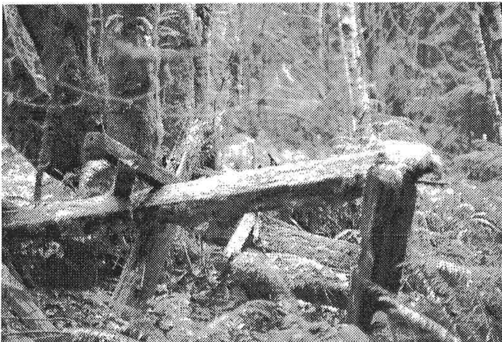
L1-6 Collapsed structure at Manganese, segment 10
