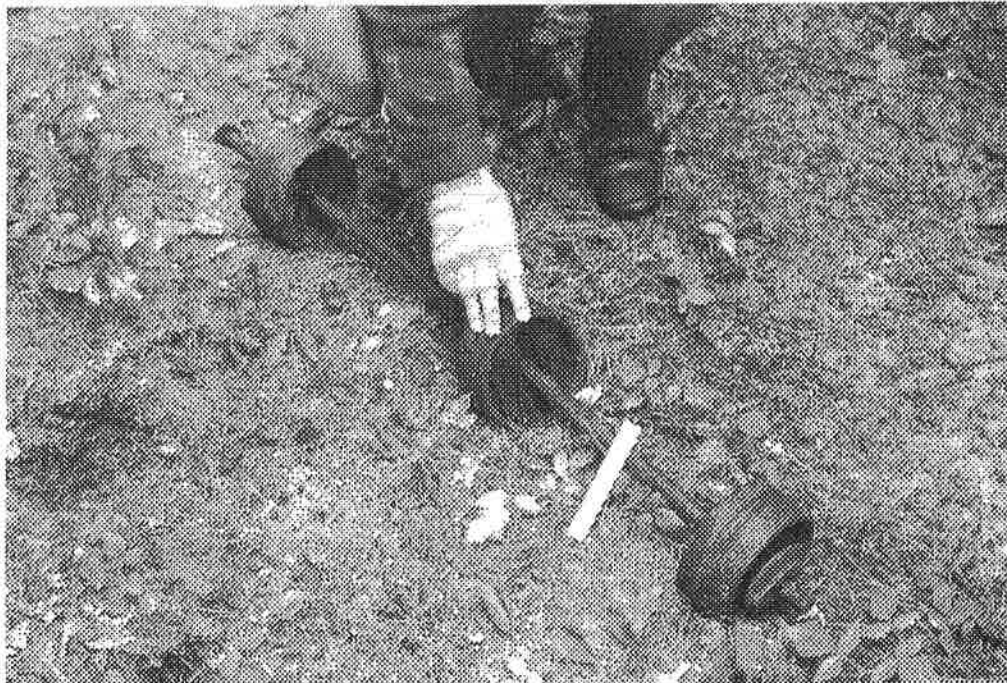
W2-13 Steel rod with castings from Howe truss. Segment 14
