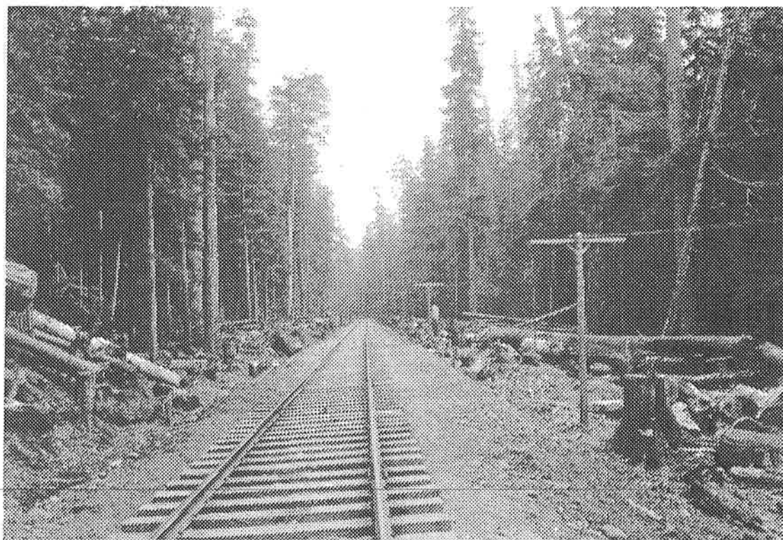
View of grade with telephone lines in place #38055
