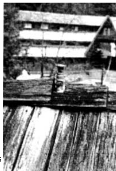
Small dormer, west side. Note the damage.
