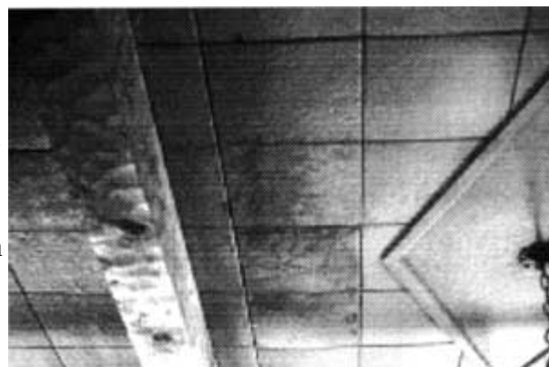
Water damage at the lobby ceiling.
