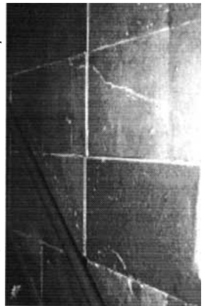
Abrasion damage at the stair.
