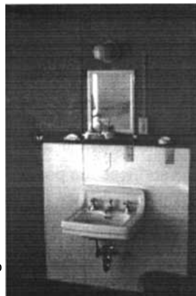
Painted sink surround, 6th floor.
