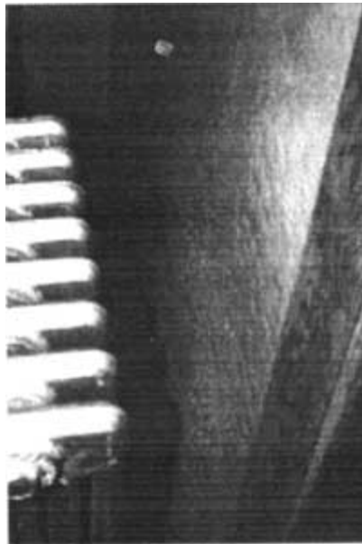
Glaze damage behind radiator.
