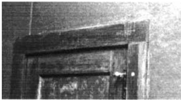
Glaze slopped onto door trim.
