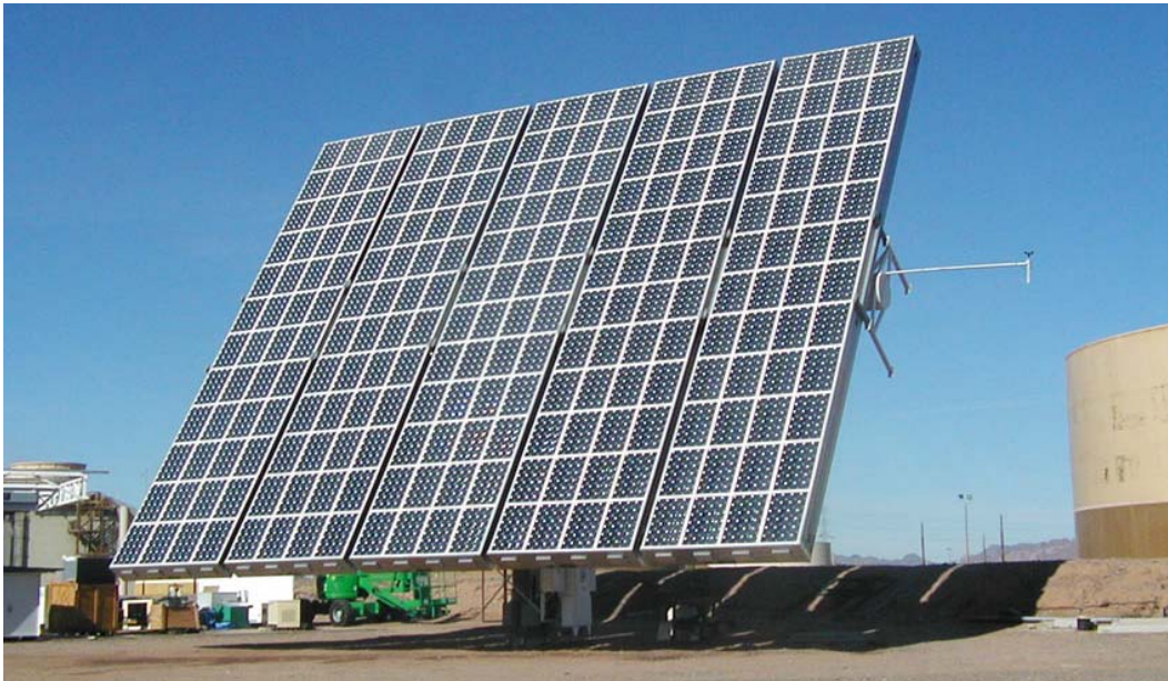
Fig. 15: An Amonix concentrating photovoltaic system.
