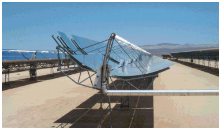
Fig. 14: Solar trough array.
