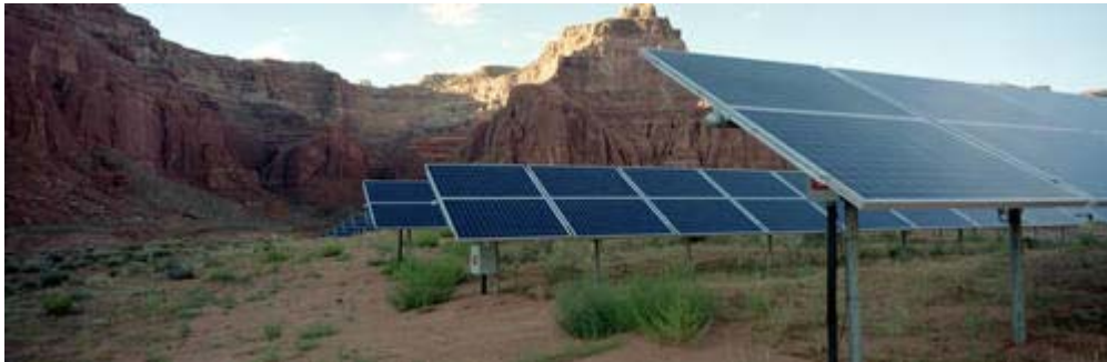
Fig. 16: Solar array at Glen Canyon National Recreation Area.
