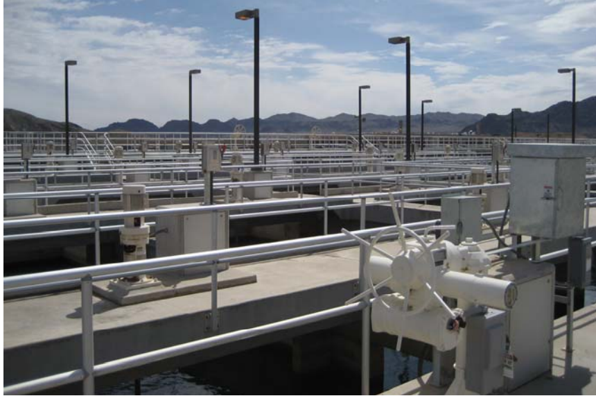
Fig. 32: Flocculation basin at the SNWA pumping station.
