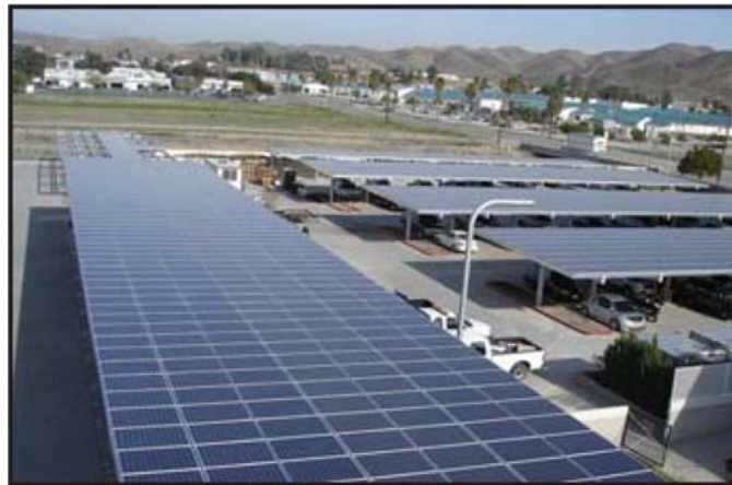
Fig. 40: Elsinore Valley Municipal Water District carports.
