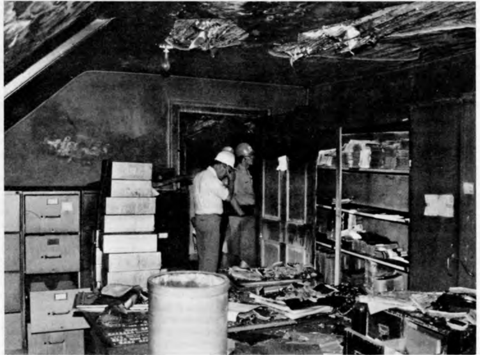
Acting Superintendent James D. Young (on right) and Safety Officer John J. Longworth examine interior of the visitor center at Harpers Ferry NHP, W. Va., which was heavily damaged by fire May 20. The visitor center will be closed indefinitely; and temporary visitor facilities have been established at the park
