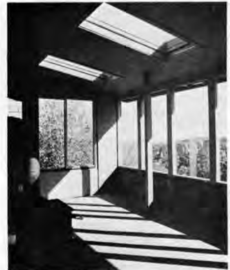
Nearing completion, the interior of the solar greenhouse at Colorado NM. The woodstove serves as a back-up on overcast days.
