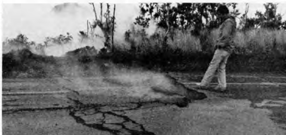
Earthquakes through a fault zone caused road damage in Hawaii Volcanoes NP. The earth steamed and the roadway dropped nearly a foot.
