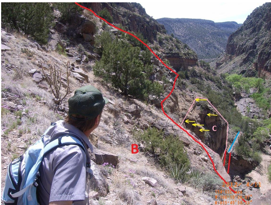
Figure 5 – View, looking downstream, from center of coarse debris fan 'B.' Blue line is existing trail. Two parallel red lines show destroyed section of trail. Parallel yellow arrows show vertical cracks on slope immediately above trail. Pink zone labeled 'C' shows wedge of Maar bedrock that could fail at any time.
