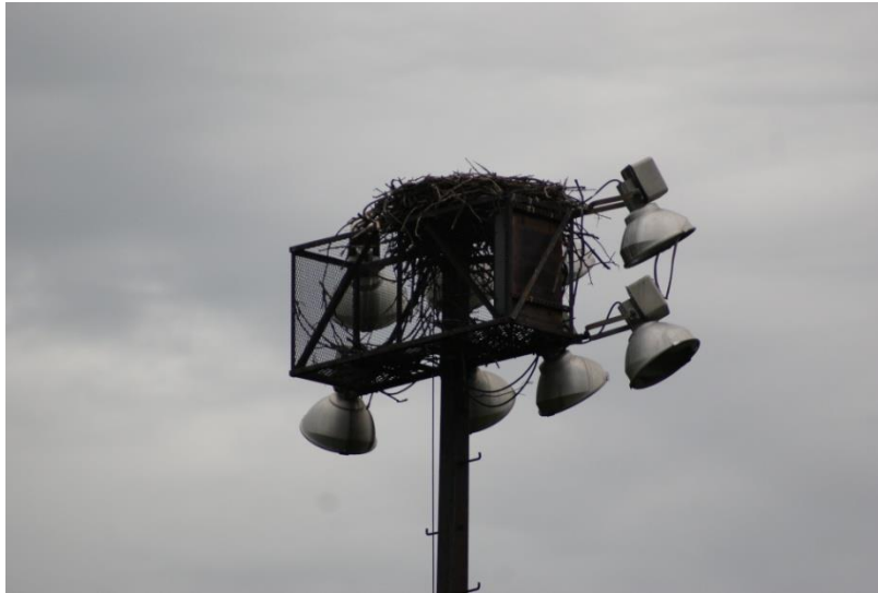
Osprey ( Pandion haliaetus ) nest in stadium lighting tower near Kenilworth Aquatic Gardens.
