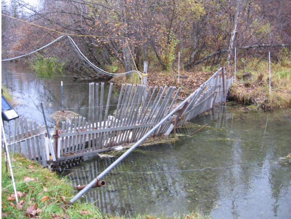
Figure 2. Weir damage from heavy leaf load, 2012.
