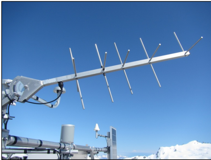
Figure 5. Chigmit Mountain RAWS – Missing tines on GOES antenna.
