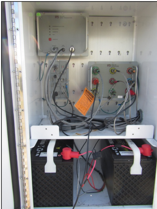
Figure 19. Fourpeaked RAWS – Inside of instrument enclosure after maintenance.
