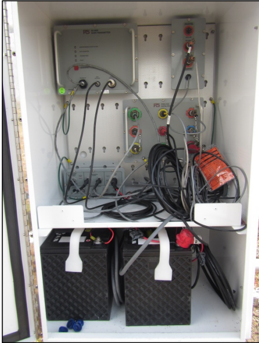
Figure 11. Coville RAWS – Instrument enclosure after maintenance.
