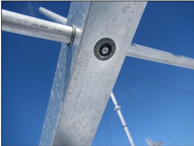
Figure 25. Harding Icefield RAWS – GOES antenna tine broken off inside antenna.
