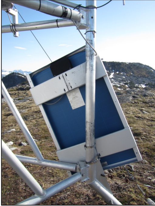
Figure 33. McArthur Pass RAWs – Three out of four hose clamps used to mount the solar panel had broken.
