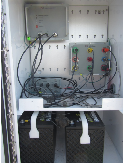
Figure 35. McArthur Pass RAWs – Inside of instrument enclosure after maintenance.
