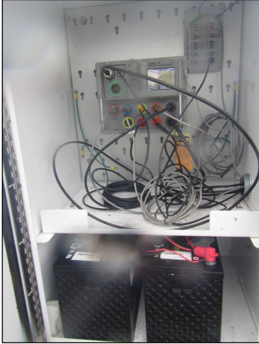
Figure 42. Pedersen Lagoon RAWS – Inside of instrument enclosure after maintenance.
