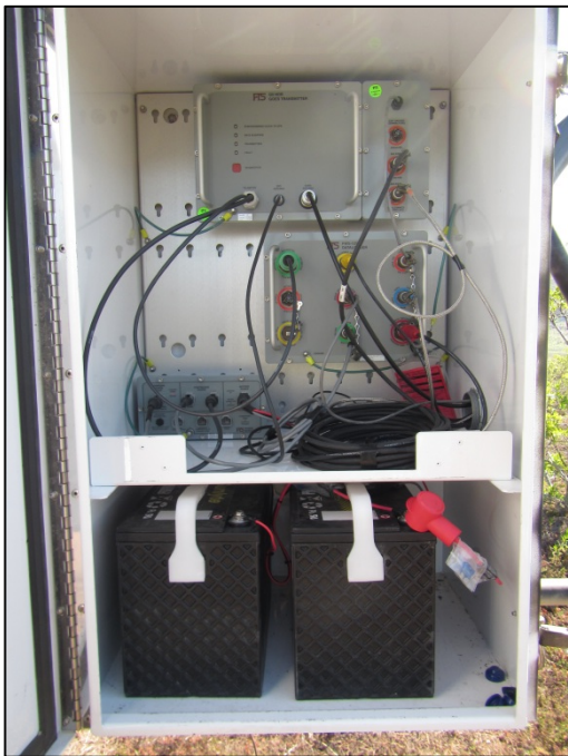
Figure 61. Three Forks weather station – Inside of instrument enclosure after maintenance.
