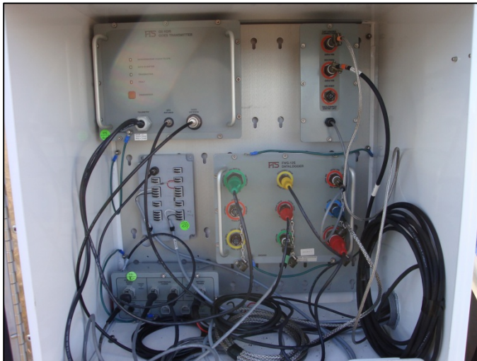
Figure 49. Pfaff Mine RAWS – Inside of instrument enclosure after maintenance. The soil temperature sensor and SDI-AM are not plugged into the data logger.
