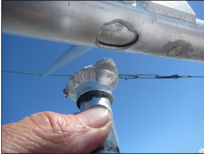
Figure 2. Chigmit Mountain RAWS – Broken weld on spreader bar that supports guy-wires for the wind sensor mast.
