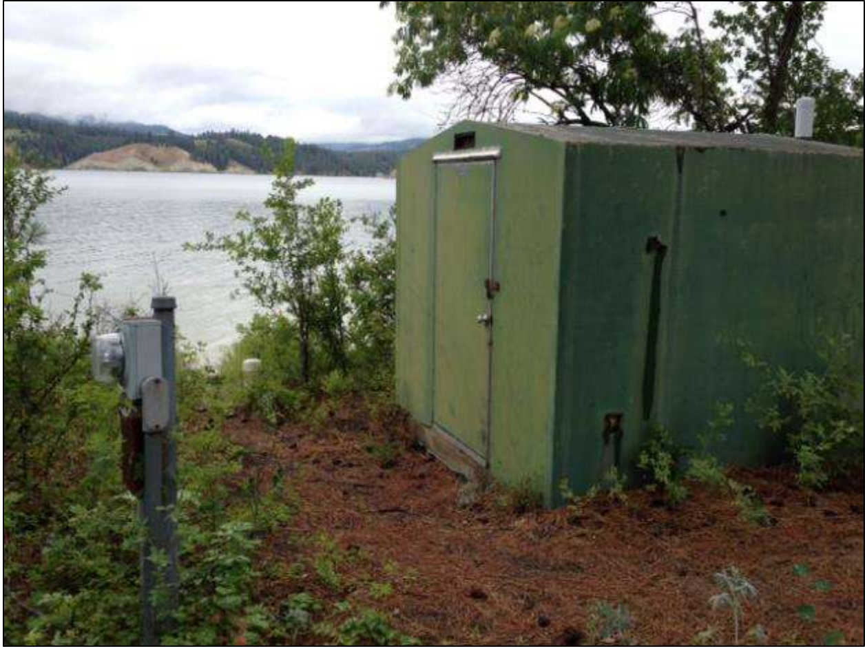
Figure 3. Hunters campground Well No. 1 is inside the green building. The well is 30 feet from the lake.
