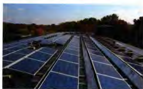
Solar panels installed on the flat roof.
