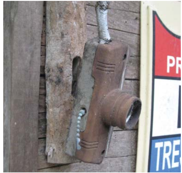
Figure 14 , Early Bakelite Corporation light fixture mounted to the south side of the front entrance door.
