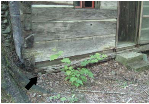
Figure 28, Southeast corner exhibiting rot in bottom logs, both south and east elevations.
