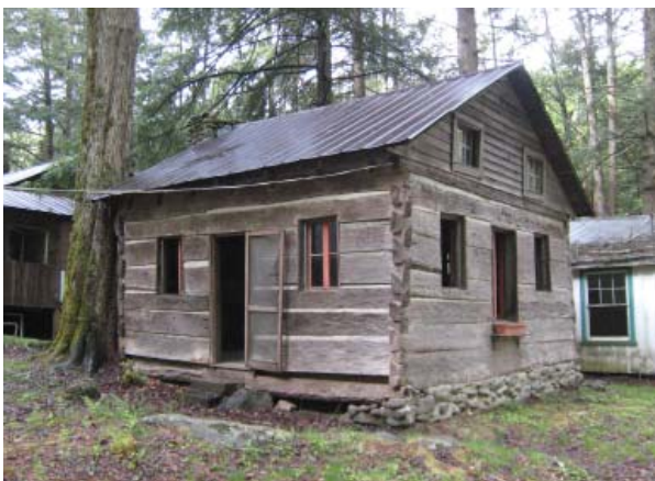
Figure 7, Northeast oblique of cabin showing partially collapsed east foundation wall.
