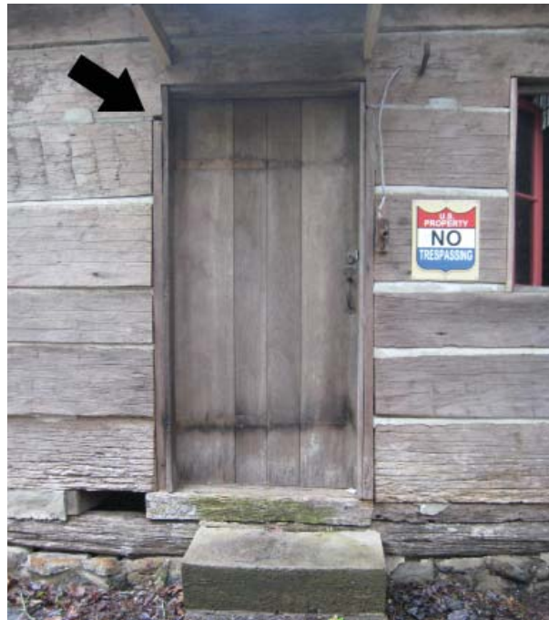
Figure 17, West elevation doorway notched for earlier, shorter and wider door.
