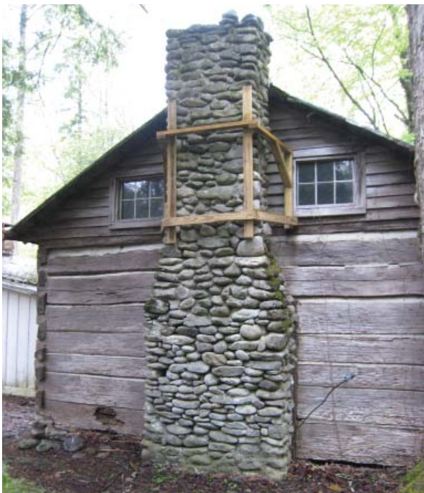
Figure 16, River stone chimney on south elevation with recently added frame for support.
