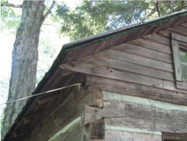
Figure 12 , An electrical wire connected the Mayo Servants' Quarters to the Trentham Cabin fuse box, which in turn connected to the Mayo Cabin.
