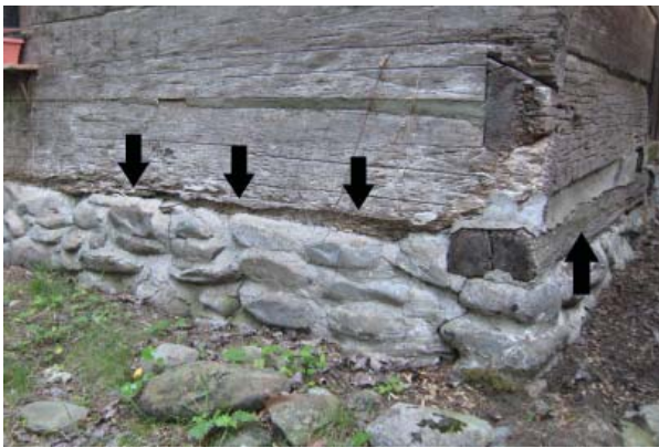
Figure 6, Northwest corner with unhewn sacrificial bottom log on west elevation (right) and rot in hewn bottom log of north elevation (left).
