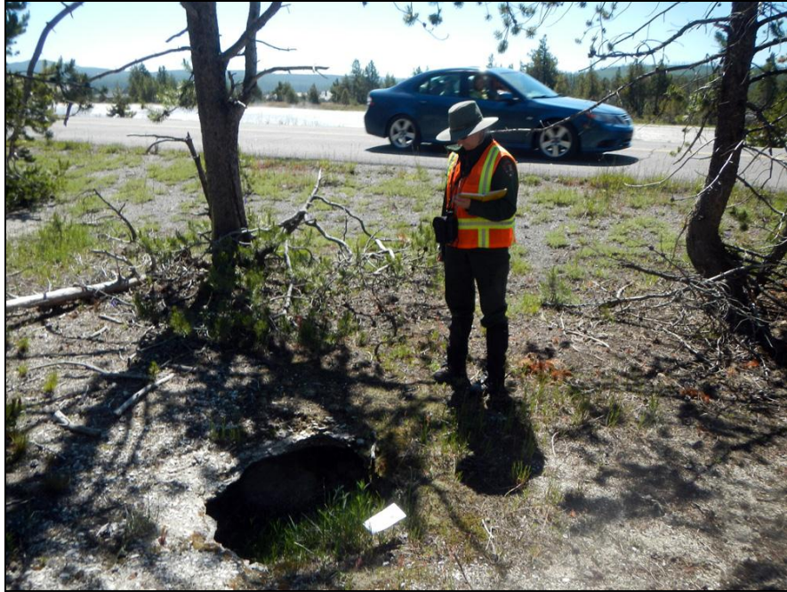
Figure A2. Photograph of hydrothermal vent “C”. The two-lane service road is visible in the background. View to the south on 2 July 2014.
