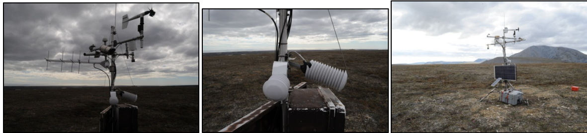
Figure 16. Mt. Noak, June 4, 2015. Site shown before (left) and after (right) repairs. The AT-RH radiation shields (middle) were bent horizontally, presumably by musk oxen.
