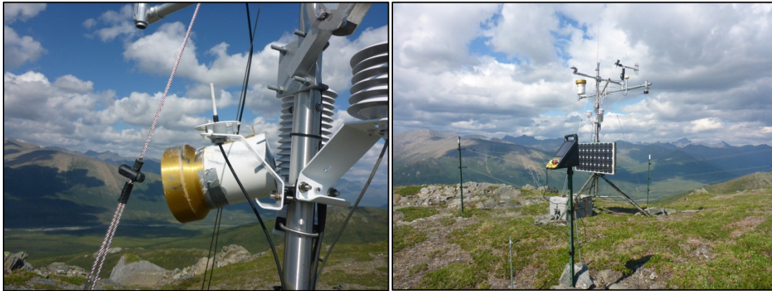
Figure 2. Chimney Lake, July 1, 2015 before (left) and after (right) maintenance. Upon arrival at the site the RG-TB and 109-L AT radiation shield were damaged.
