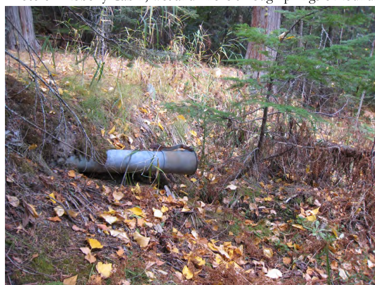
Photo 8. Pipe above slope from Moberly Cabin diverting spring water
