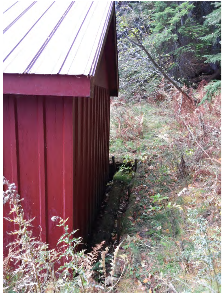
Photo 18. Foundation of Fox Cabin; stream flows underneath
