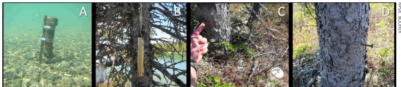
Figure 15. The Solinst level logger (A) and baro logger (B), as installed at the Lake Clark outlet on June 3, 2014. A survey was completed on that date to establish the elevation of the level logger relative to existing reference points, RP1 (C) and RP2 (D). Note that the benchmark monument is located near the base of the tree holding the RP1 nail (C).
