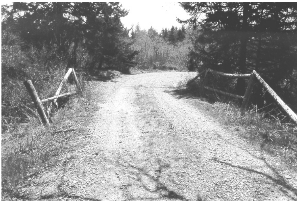
Deteriorating rustic-style timber railing along Schoodic Head Road (OCLP, 2000).
