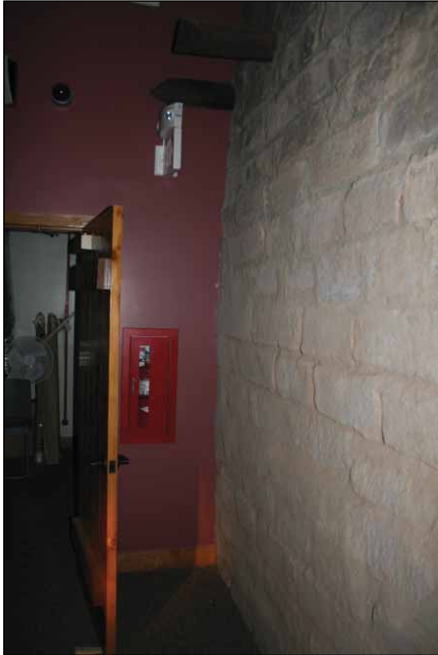
Figure 7. Northeast interior wall of theater addition showing profile of original exterior portale wall. Note apparent bulging.
