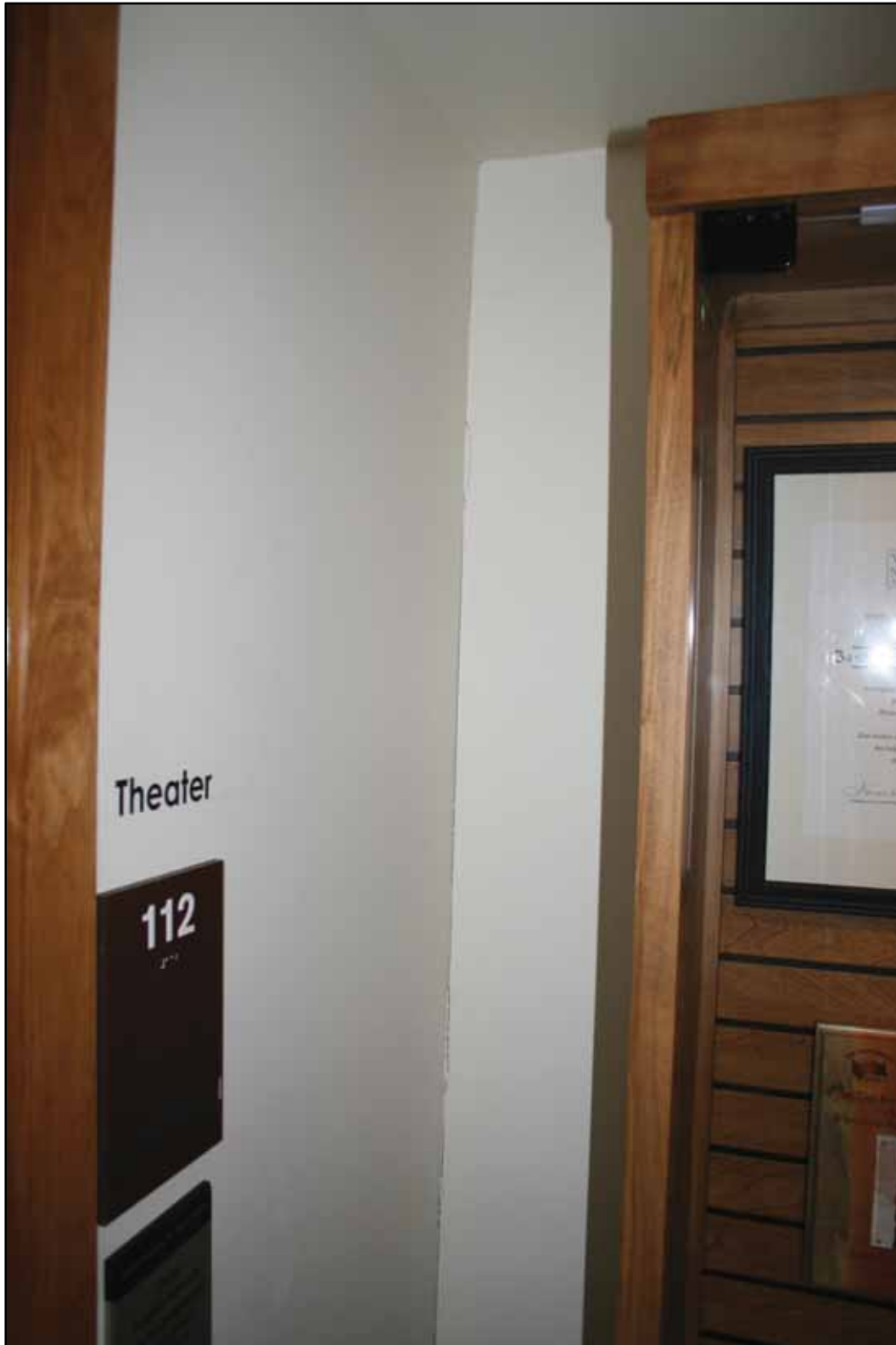
Figure 15 Photo of hall (Room 119) wall intersection with Theater (Room 112) showing minor separation at corner.
