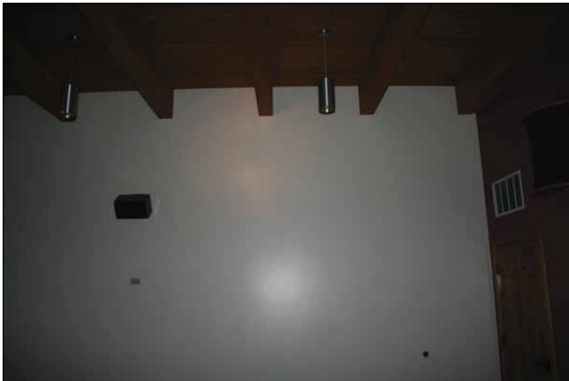
Figure 10. Southeast end of southwest wall of theater addition.
