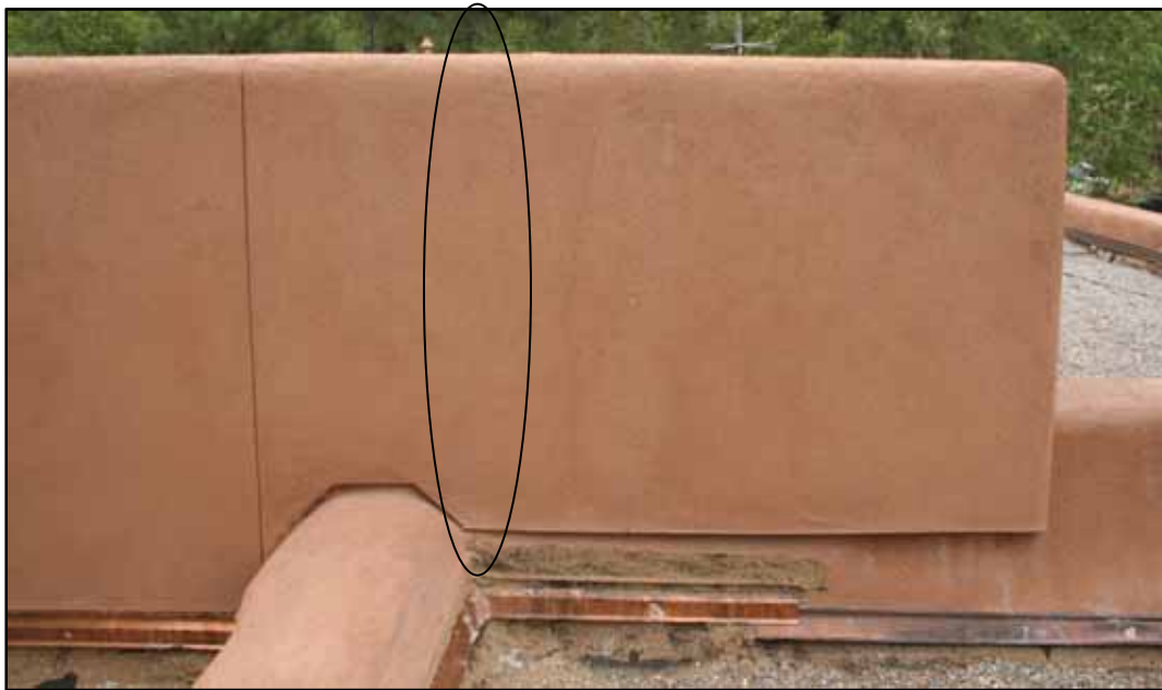
Figure 4. Southeast wall of Theater showing minor cracking.
