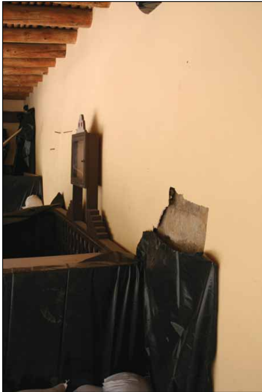
Figure 6. Plaster loss on northwest wall of Portale.
