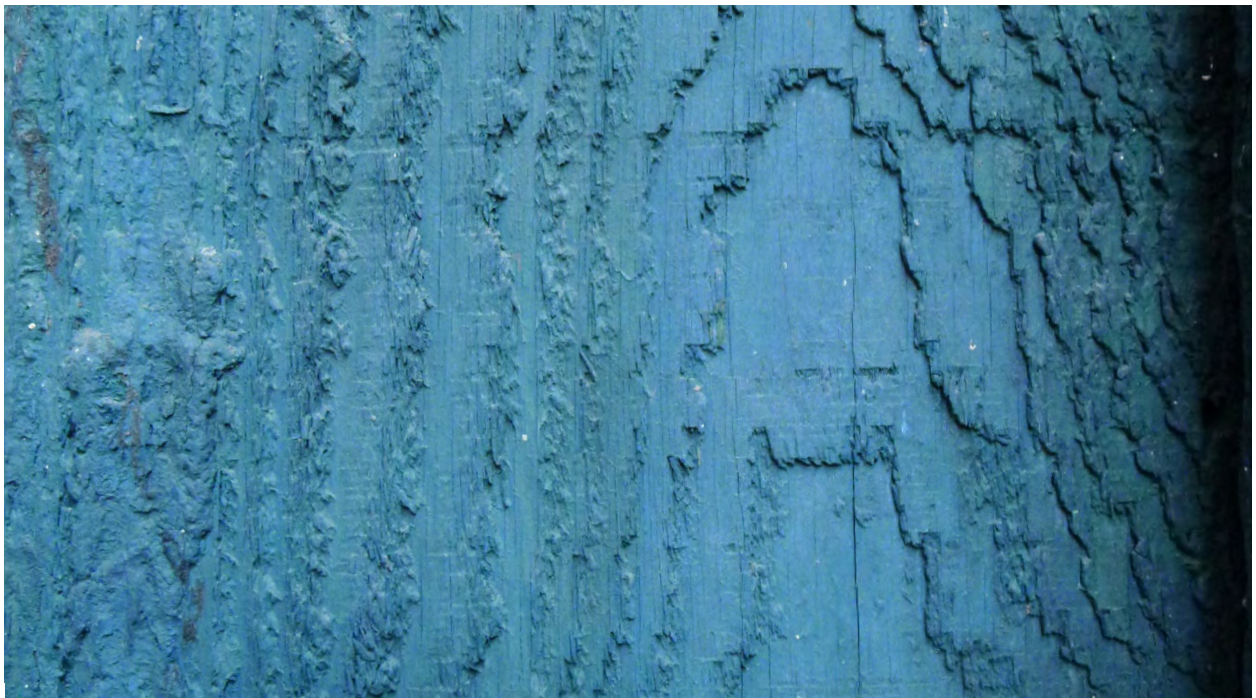
Figure 3: Rough painted surface of the wood siding.
