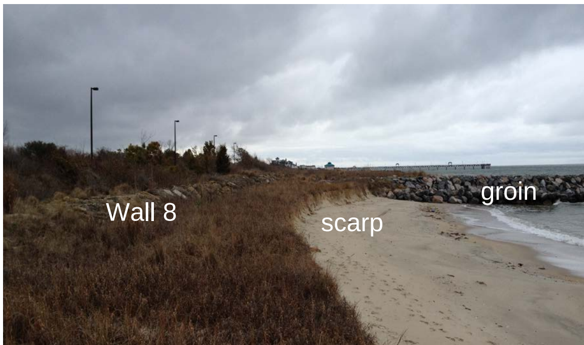
Figure 2. Shoreline downdrift of the middle groin in Groin Field 1, showing erosional scarp and concrete riprap in Wall 8 at left.
