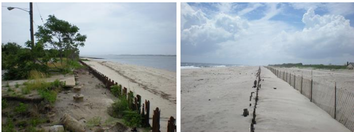
Figure 3. Deteriorated bulkheads at Gateway considered for elimination using post Hurricane Sandy rehabilitation funds. Left panel is Wall 2 at Aviation Rd. and right panel is Wall 28 at Ft. Tilden (Figure 20, Table 7, Appendix A).
