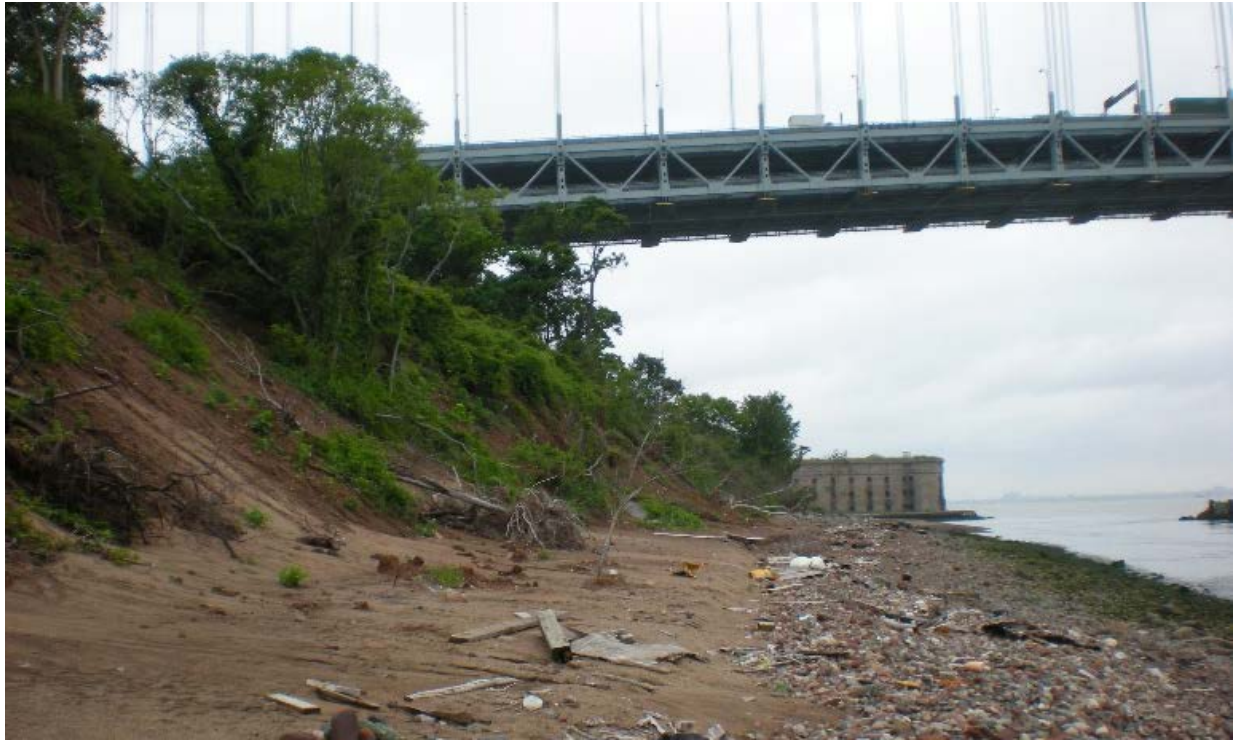
Figure 23. Eroding bluff at Battery Hudson, Staten Island Unit, showing protection provided by gravel at the base and delivery of sediment from the bluff face.
