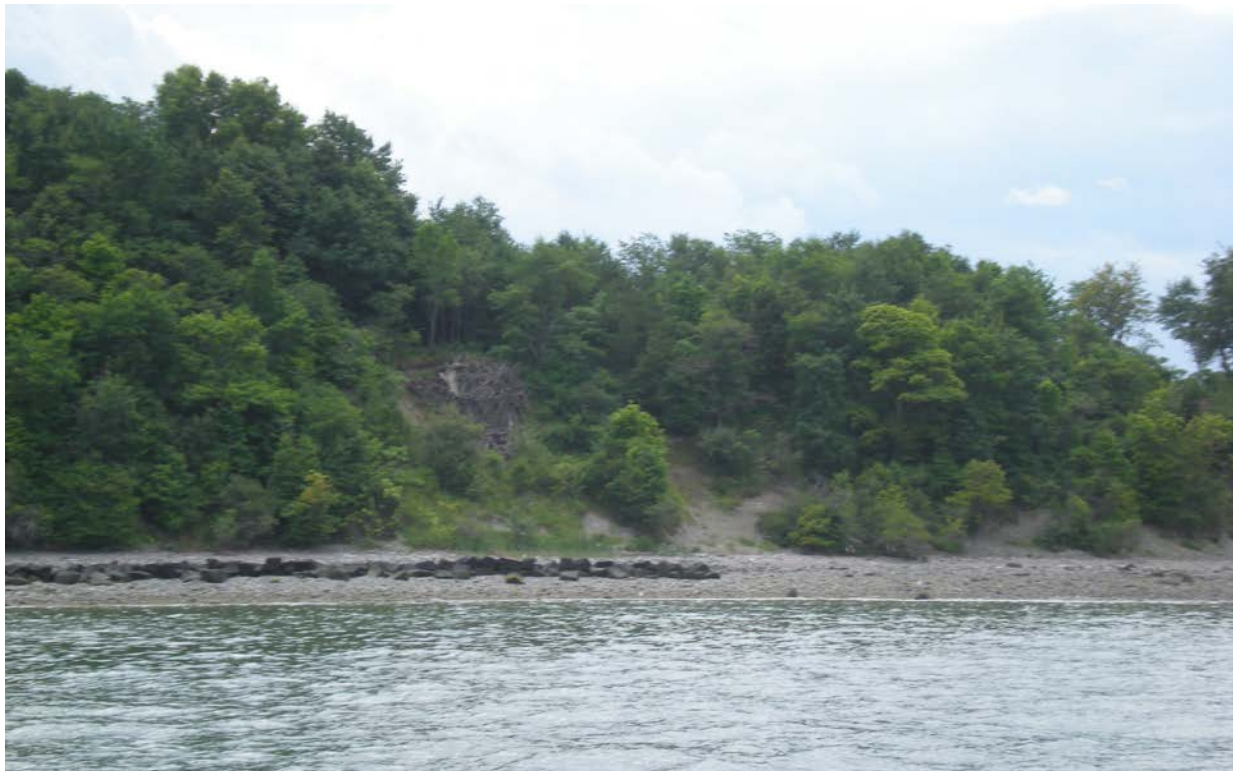
Figure 13. Thompson Wall 1 (Figure 11E), showing greater erosion on the unprotected bluff on the south (right) side of the wall than on the bluff landward of the wall.
