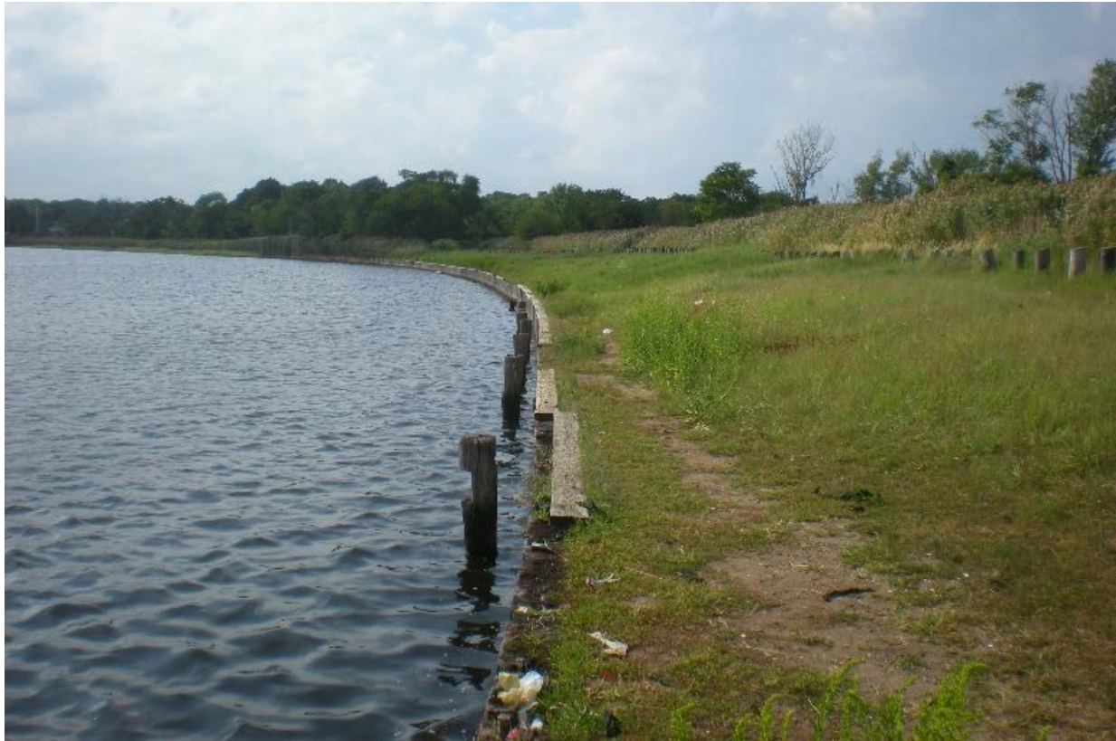
Figure 24. Deteriorating bulkhead near center of Wall 8, Great Kills Park area, Staten Island Unit.
