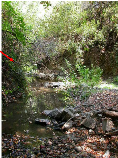
Photo 11: Looking downstream at toe of NPS bank below gravesite
