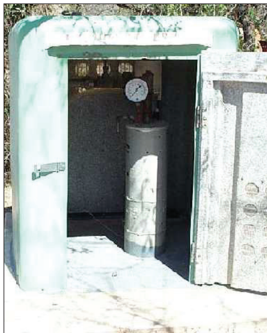
Figure 3-4. The Mission unit's water-supply well, monitored manually (via sounding tape) since 1960.
