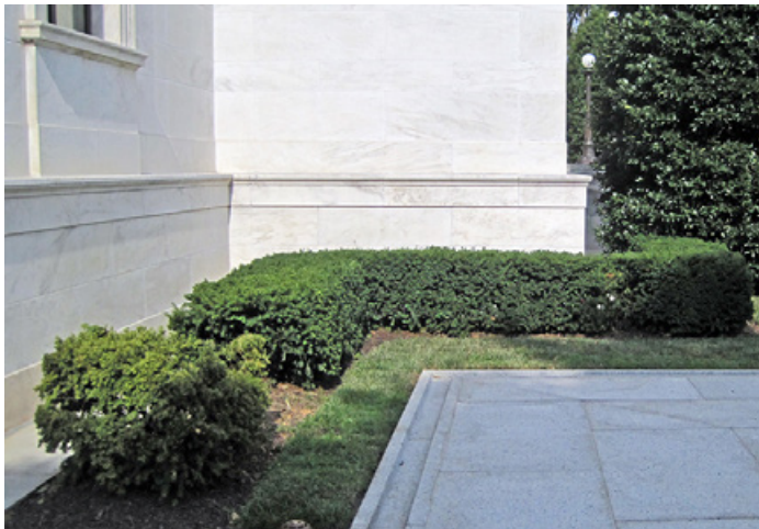
Figure 38 – Yews lining building and grass strip in front. The end of the yew hedge is in poor condition with a gap in planting.
