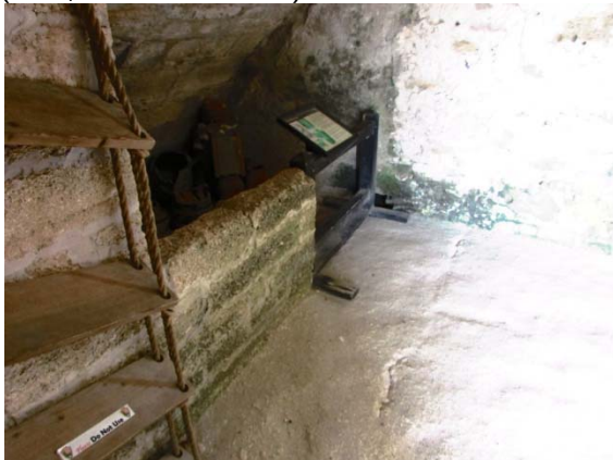
Photo E-7: Crack in tabby floor topping (2016, Faisant Associates).
