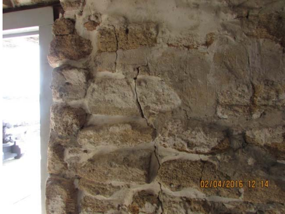
Photo C-3: Wall crack, west side of doorway (2016, Faisant Associates).
