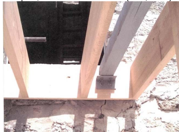
Photo B-13: Wall crack at beam seat connection, 1998 stair reconstruction (1998, FOMA).
