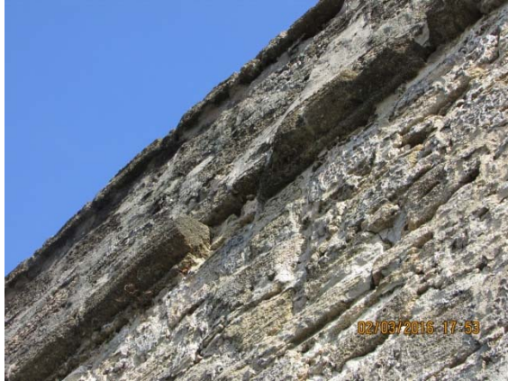
Photo A-1: Cordon course deterioration, at north tower wall (2016, Faisant Associates).
