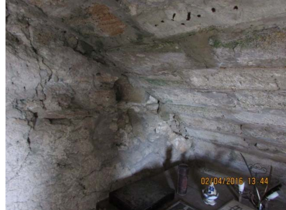
Photo E-4: Wall cracks, northeast corner (2016, Faisant Associates).
