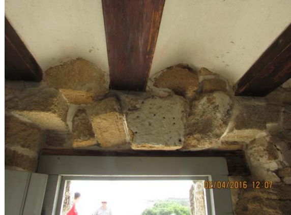
Photo C-4: Crack at door head (2016, Faisant Associates).
