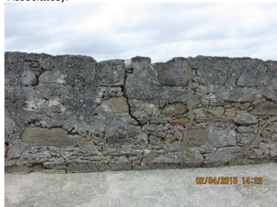
Photo A-12: Crack in north tower parapet wall (2016, Faisant Associates).
