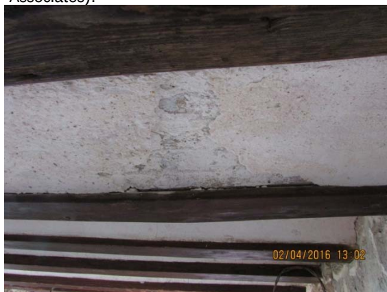
Photo D-3: Deflecting floor joist and delaminated tabby ceiling vault (2016, Faisant Associates).
