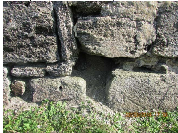
Photo A-4: Void at base of north scarp (2016, Faisant Associates).
