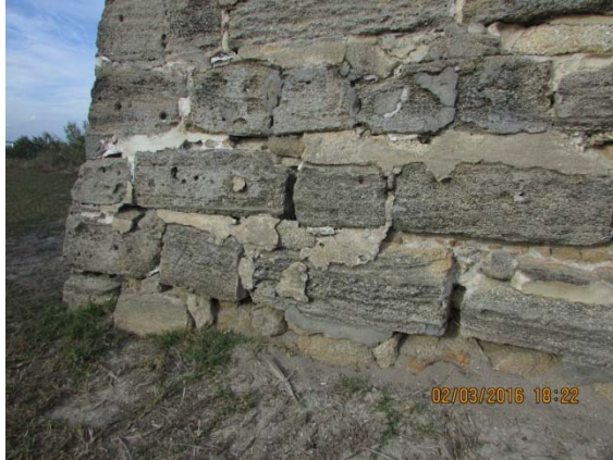
Photo A-5: Coquina erosion at northwest scarp (2016, Faisant Associates).
