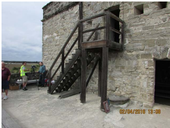
Photo A-11: South tower wall cracks (2016, Faisant Associates).
