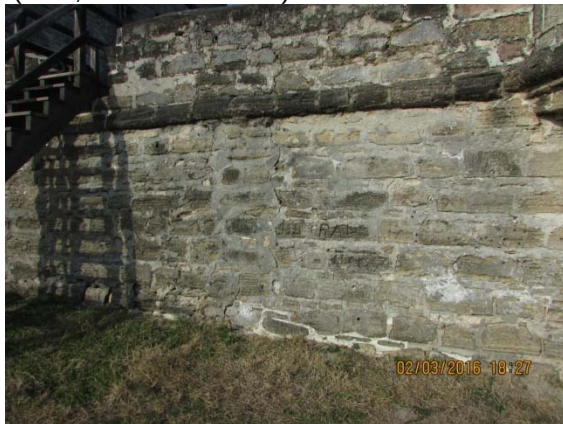
Photo A-7: Settlement crack at west scarp (2016, Faisant Associates).
