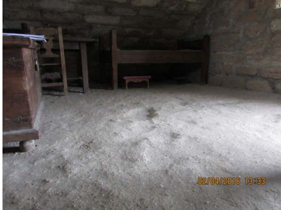
Photo E-3: Deteriorated second floor tabby topping (2016, Faisant Associates).
