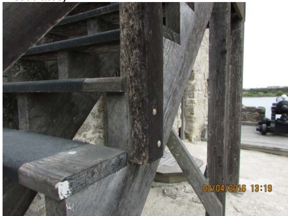
Photo B-9: Stair rail post connection (2016, Faisant Associates).
