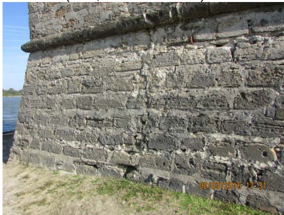
Photo A-3: Crack at north scarp (2016, Faisant Associates).
