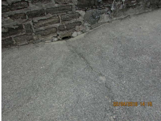
Photo F-1: Roof tabby crack at scupper (2016, Faisant Associates).
