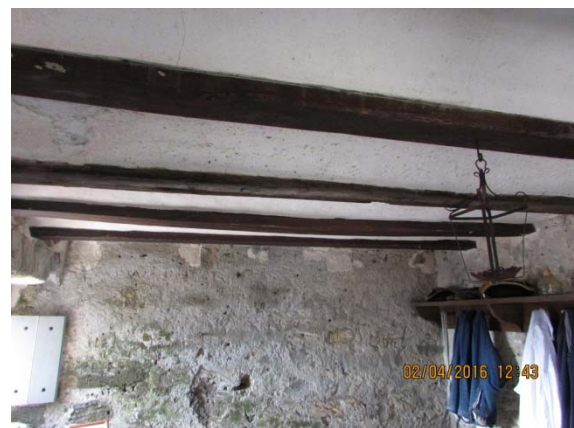
Photo D-2: Deflecting floor joist (2016, Faisant Associates).
