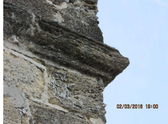
Photo A-2: Cornice erosion at southeast tower corner (2016, Faisant Associates).
