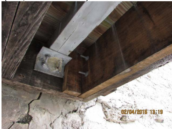
Photo B-12: Wall crack at beam seat connection (2016, Faisant Associates).
