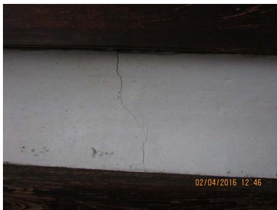
Photo D-1: Crack in ceiling vault (2016, Faisant Associates).
