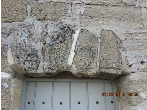
Photo A-9: Second floor door head crack (2016, Faisant Associates).
