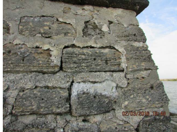
Photo A-10: Coquina erosion at portland cement mortar repointing at south scarp (2016, Faisant Associates).
