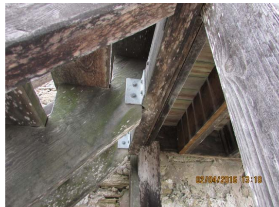
Photo B-8: Biological growth on stair framing (2016, Faisant Associates).
