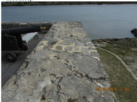
Photo A-13: Cracks in parging at top of south scarp (2016, Faisant Associates).
