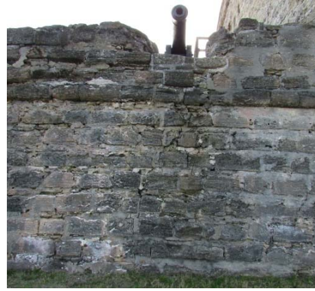
Photo A-6: Crack at east wall embrasure (2016, Faisant Associates).
