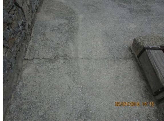
Photo F-2: Roof tabby crack at hatch opening (2016, Faisant Associates).
