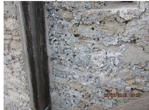
Photo A-8: Coquina erosion at south tower wall (2016, Faisant Associates).
