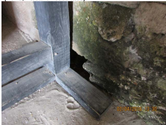
Photo E-5: Void in north wall and biological growth (2016, Faisant Associates).
