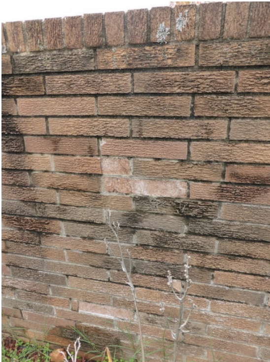
FIGURE 312. The brick wall exhibits evidence of biological growth and discoloration.
