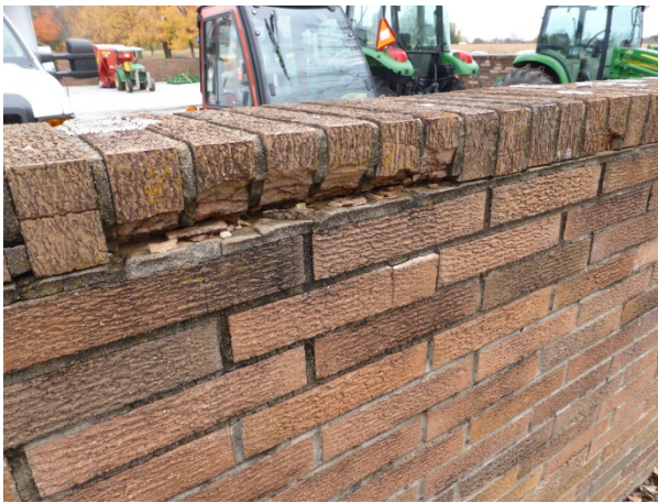
FIGURE 142. Detail of the deteriorated masonry wall surrounding the maintenance yard.
