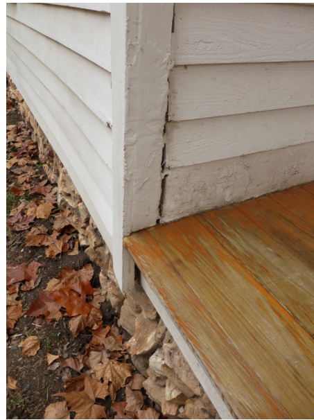
FIGURE 131. Detail of the junction of the front porch and the main house showing the separation of siding and porch elements caused by settlement and other movement.
