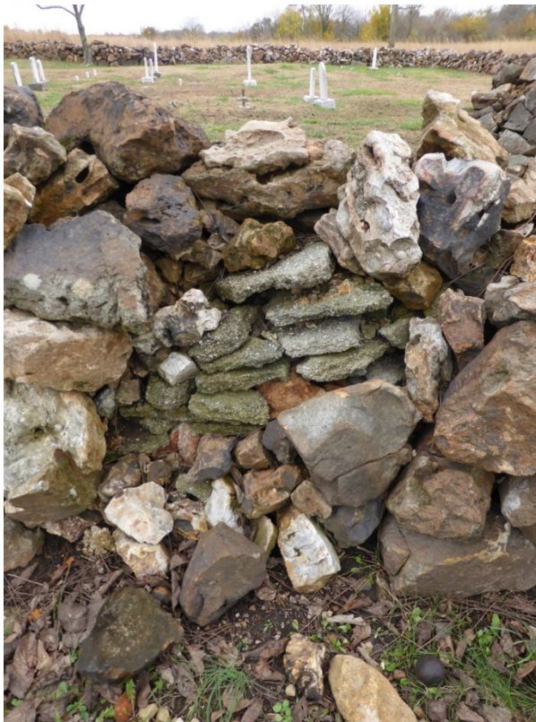
FIGURE 297. Stones that have become dislodged or displaced have been placed on top of the wall as a repair measure. The wall currently requires a comprehensive restoration to reflect its original design.
