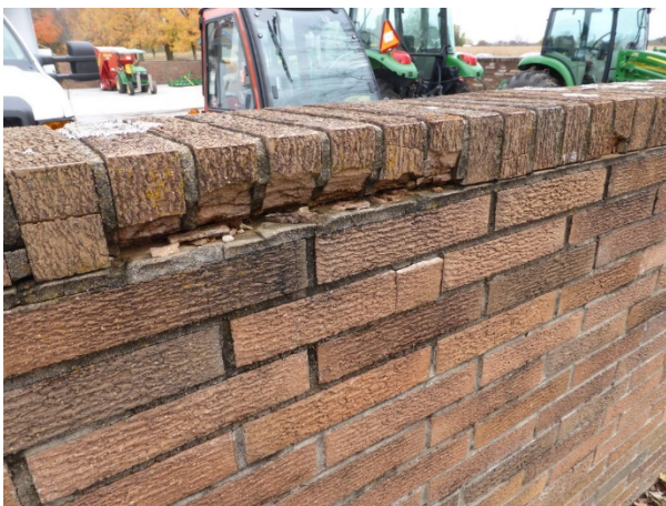
FIGURE 313. Portions of the wall are in need of repair.
