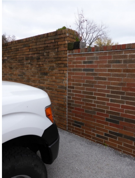
FIGURE 314. One part of the wall appears newer. The brick exhibits fewer problems with biological growth. The mortar is also a different color and less deteriorated.
