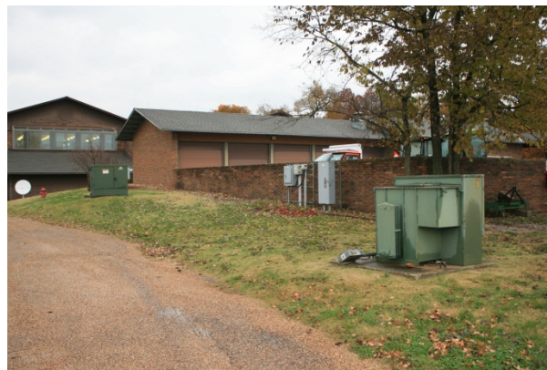
FIGURE 173. Electrical boxes west of the maintenance yard wall.
