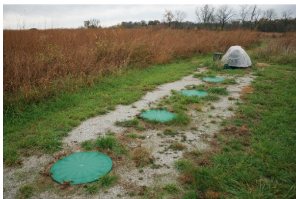
FIGURE 172. Above ground portions of the septic system.
