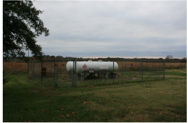
FIGURE 174. Liquid petroleum gas (propane) tanks are stored in a fenced enclosure south of housing complex.
