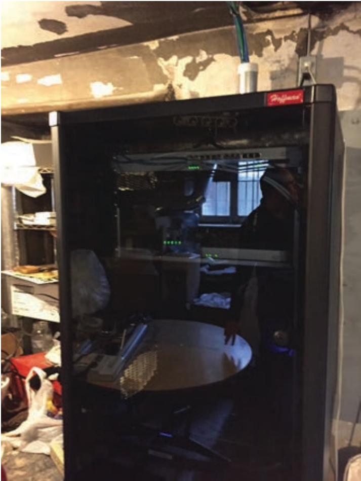
Security and data system in basement
