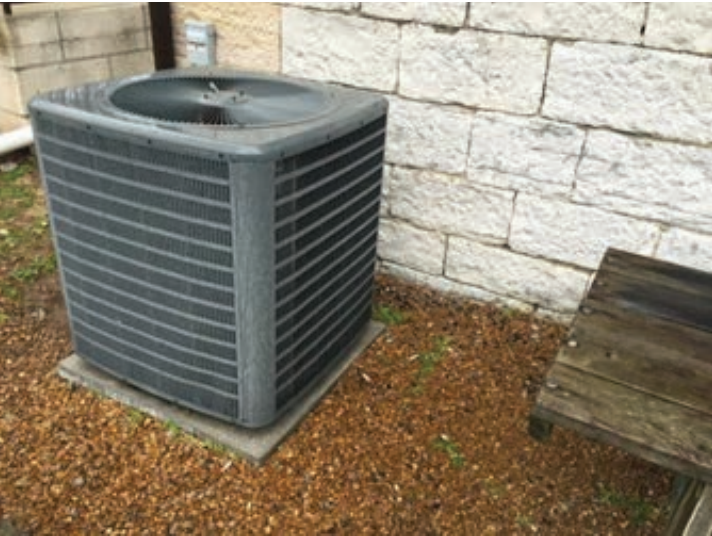
HVAC Back Ell Condensing Unit
