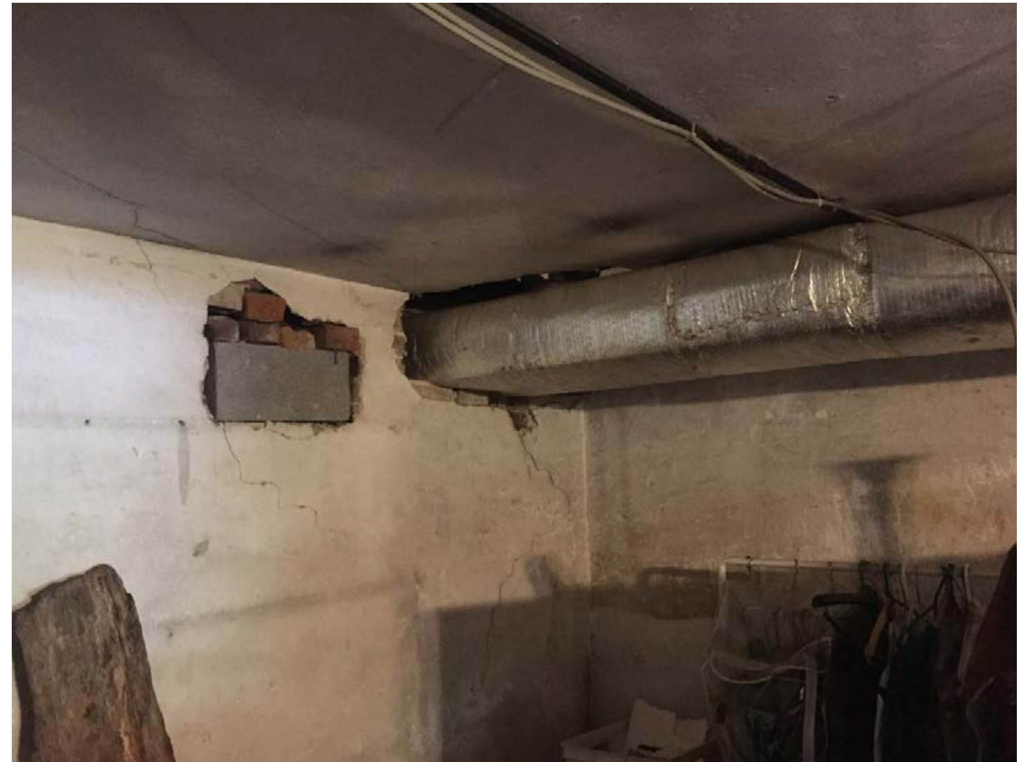
HVAC ductwork runs throughout the basement
