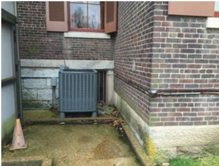
HVAC 1st floor condensing unit
