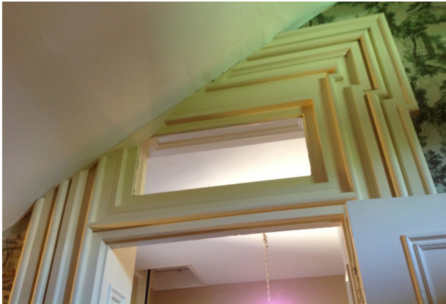
Lack of an architect is made evident in how the staircases and door transoms are mismatched
