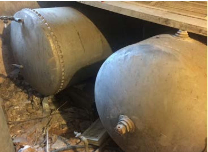
Water tanks that were once part of the radiator heat
