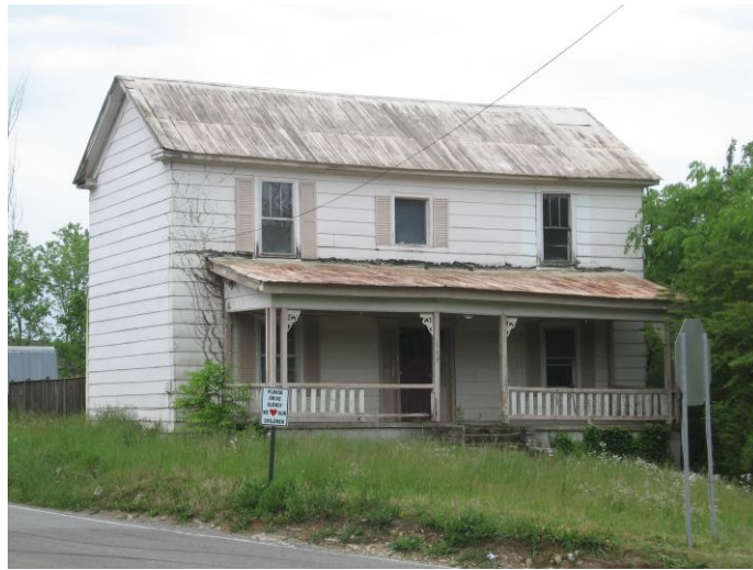
Figure 37: CP-222 at 5666 Old Middlesboro Highway.
