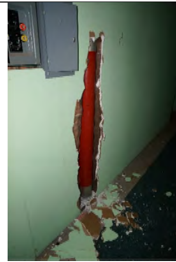
PHOTO 42: COLUMN DISCOVERED IN APT PARTITION IN FORMER BALLROOM
