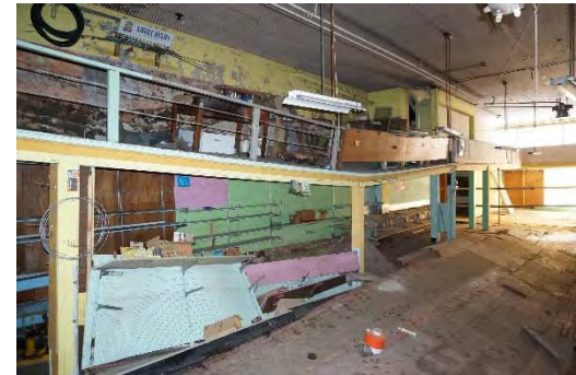
PHOTO 39: COLLAPSED MEZZANINE AND FIRST FLOOR
