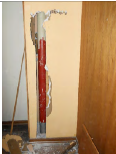
PHOTO 40: COLUMN DISCOVERED IN APT PARTITION IN FORMER BALLROOM
