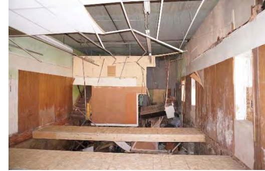
PHOTO 45: STRUCTURAL BRACING AT FIRST FLOOR LINE IN AREA OF COLLAPSED FLOOR
