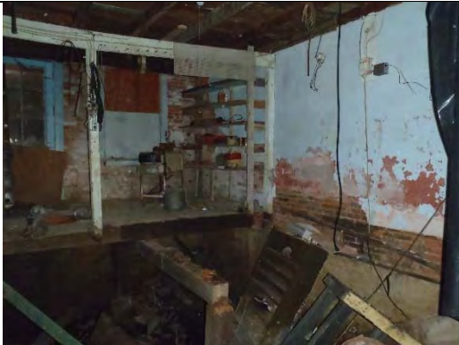
PHOTO 37: COLLAPSED FIRST FLOOR
