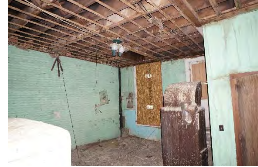
PHOTO 51: DEBRIS AND PIGEON GUANO SECOND FLOOR APARTMENTS
