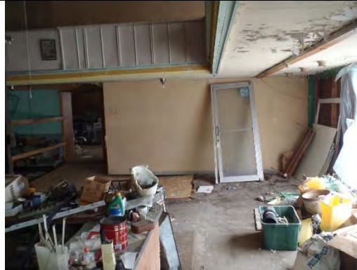
PHOTO 35: DEBRIS IN BUILDING BEFORE CLEANOUT
