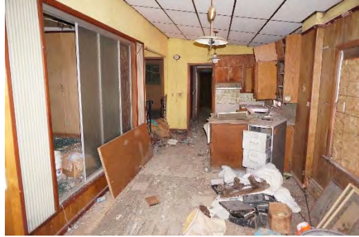
PHOTO 49: DEBRIS AND PIGEON GUANO SECOND FLOOR APARTMENTS
