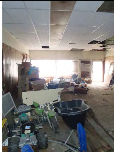
PHOTO 32: DEBRIS IN BUILDING BEFORE CLEANOUT
