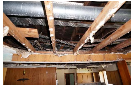
PHOTO 54: COLLAPSED CEILING FRAMING AND FINISHES IN APT AT ROOF LEAK
