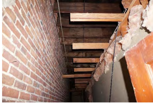
PHOTO 50: SECOND FLOOR APT CEILINGS FRAMED LOWER THAN HISTORIC CEILING
