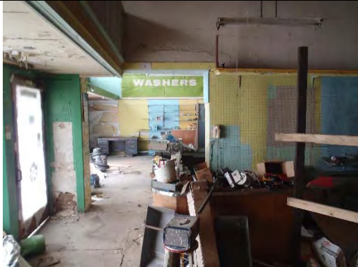
PHOTO 34: DEBRIS IN BUILDING BEFORE CLEANOUT
