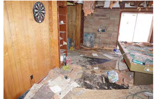
PHOTO 48: DEBRIS AND PIGEON GUANO SECOND FLOOR APARTMENTS
