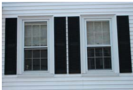
Shutters screwed to the wall are obvious fakes and should be avoided.
