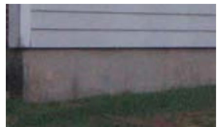
Concrete is not a traditional foundation material and should not be exposed.
