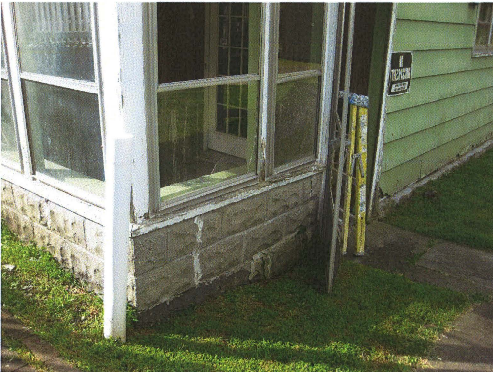
Photo #20 – Split face block knee wall at enclosed porch
