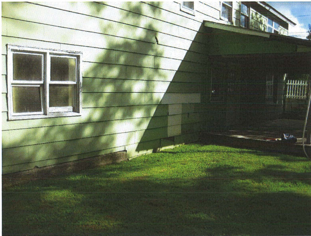
Photo #17 – Bulge in wall at rear of repurposed garage
