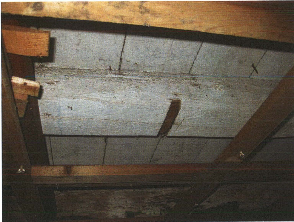
Photo #5 – Notch in second floor joists
