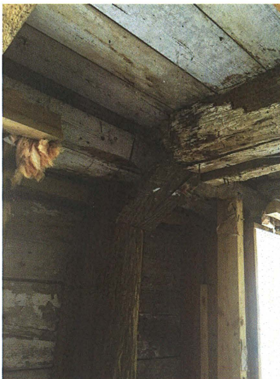
Photo #7 – Damaged and modified bearing detail at girder and supplementary posts
