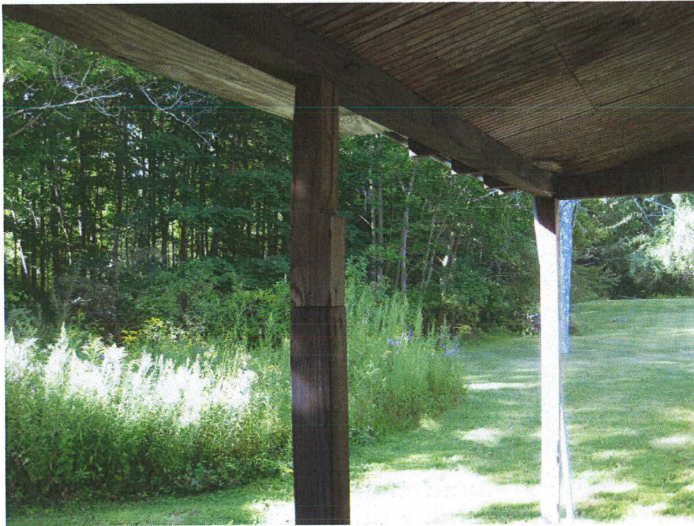
Photo #21 – Splice and notch at canopy post
