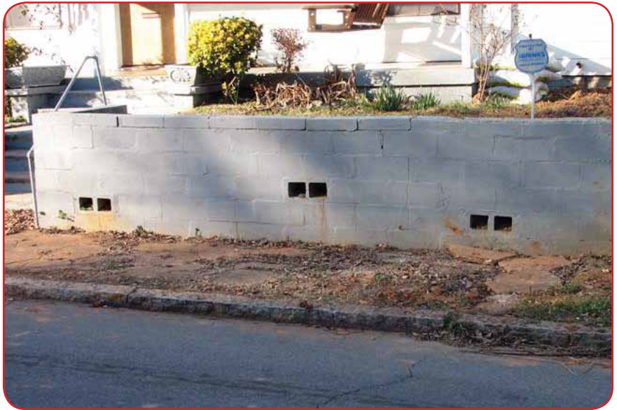
INAPPROPRIATE RETAINING WALL: INCOMPATIBLE DESIGN AND MATERIALS
