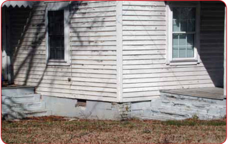
INAPPROPRIATE INFILL BETWEEN HISTORIC BRICK PIERS: INCOMPATIBLE MATERIAL NOT RECESSED
