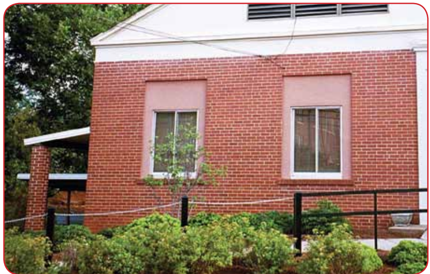
INAPPROPRIATE WINDOW REPLACEMENT: INCOMPATIBLE TYPE AND SIZE
