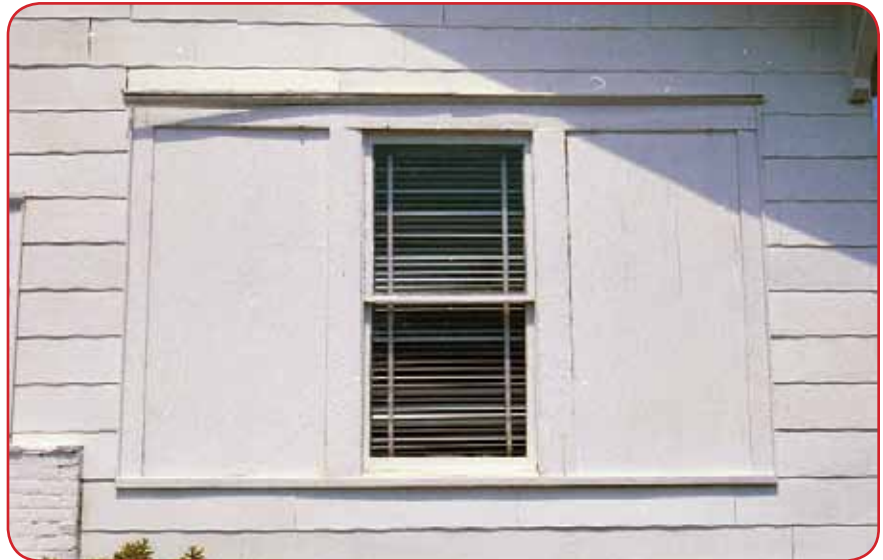
INAPPROPRIATE INFILL OF HISTORIC TRIPARTITE WINDOW
