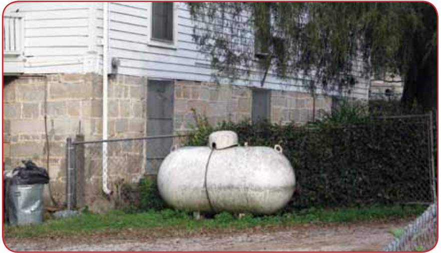
INAPPROPRIATE TREATMENT: UNSCREENED UTILITY
