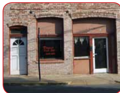
EXAMPLE OF INAPPROPRIATE TREATMENT: INCOMPATIBLE REPLACEMENT DOORS
