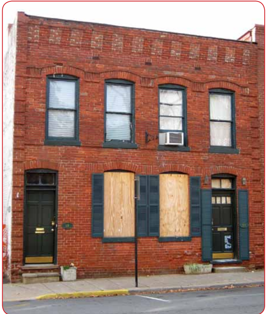
INAPPROPRIATE WINDOW ENCLOSURE
