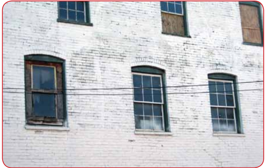
INAPPROPRIATE REPLACEMENT WINDOWS: INCOMPATIBLE SIZE, MATERIALS, AND INCONSISTENT GLAZING PATTERN
