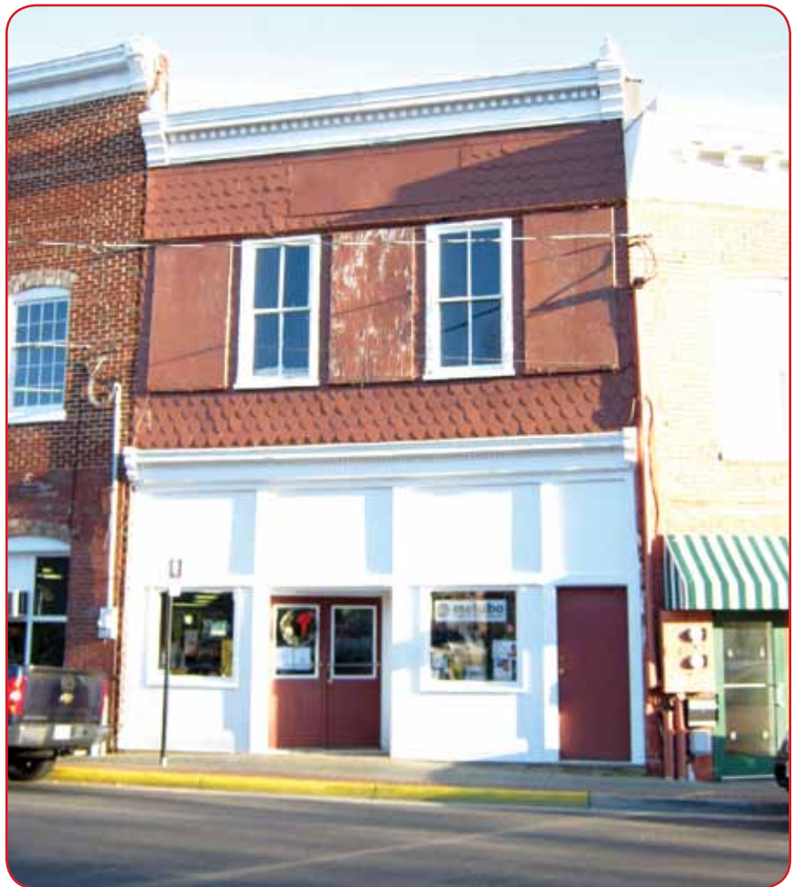
EXAMPLE OF INAPPROPRIATE TREATMENT: ENCLOSED AND ALTERED DISPLAY WINDOWS, TRANSOMS, AND ENTRYWAYS
