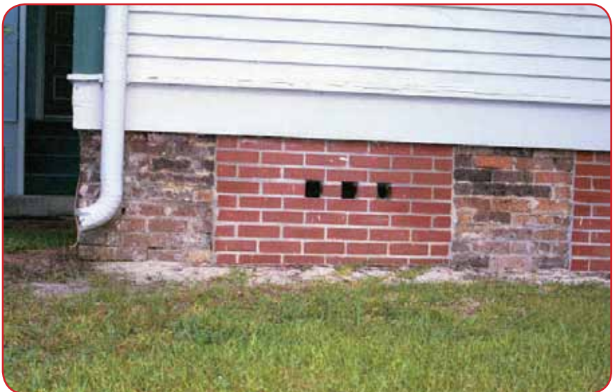
INAPPROPRIATE INFILL BETWEEN HISTORIC BRICK PIERS: INCOMPATIBLE BRICK NOT RECESSED
