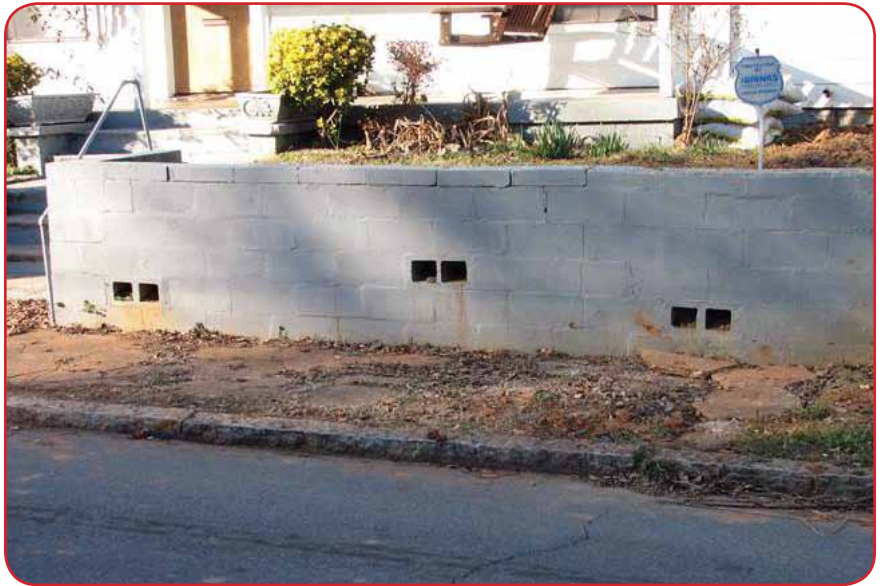
INAPPROPRIATE RETAINING WALL: INCOMPATIBLE DESIGN AND MATERIALS
