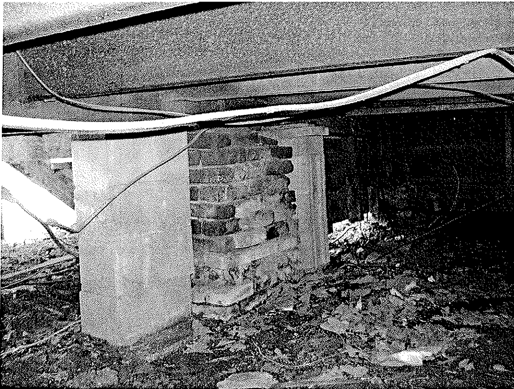
Cinder block added to stabilize deteriorating brick columns
