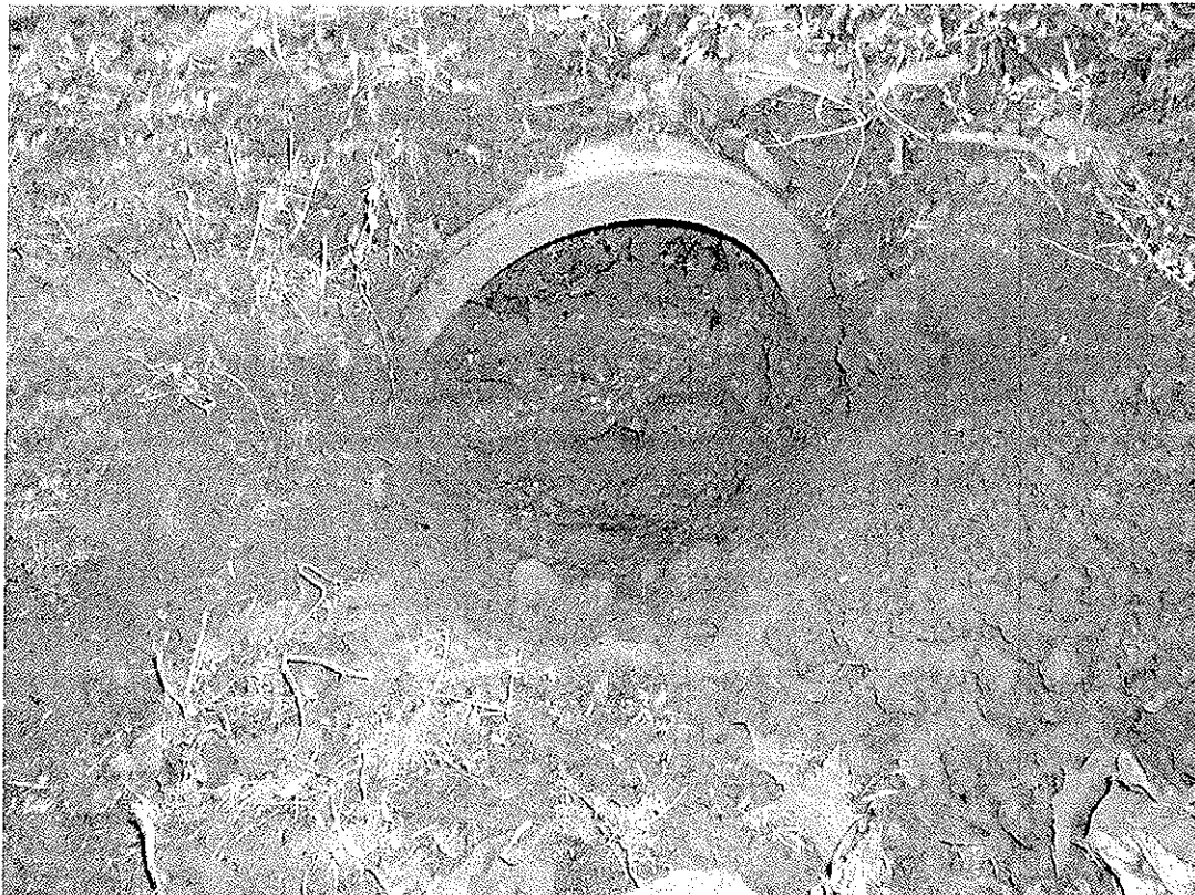
Plugged drain line
