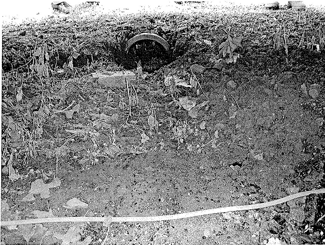
Plugged drain line
